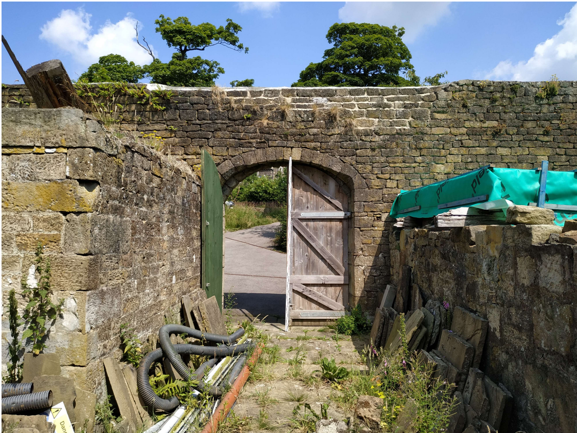
P3 Internal view of north cart entrance with remains of stone cross-walls either side
