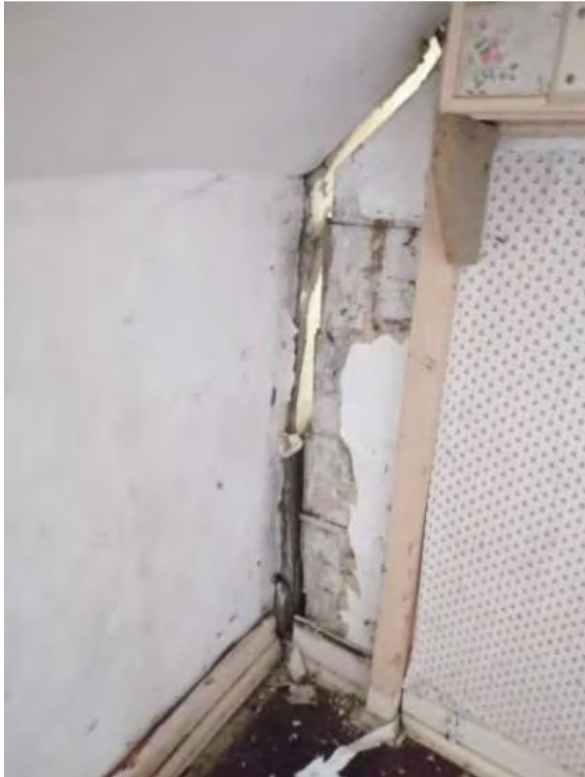
Fig 4.9 2; Movement between floor boards and wall to landing and south wall
