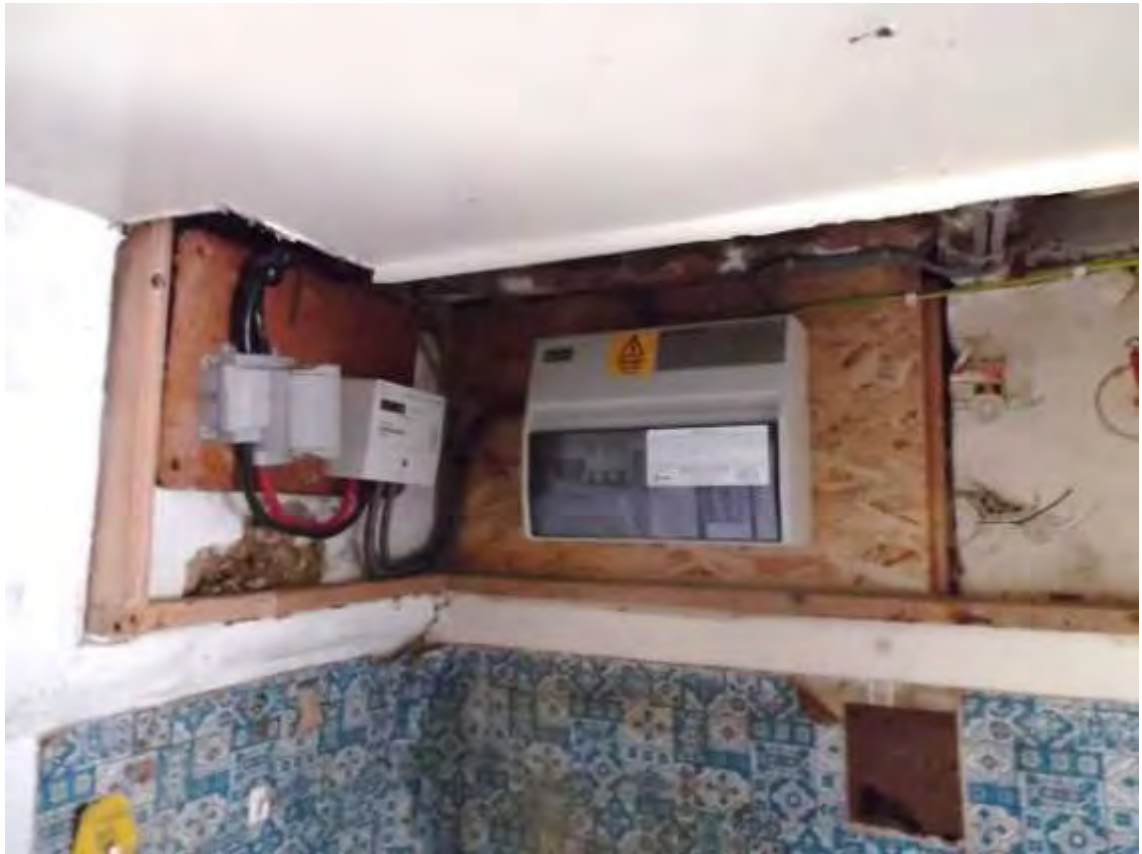
Fig 5.1; Electricity in-take board
