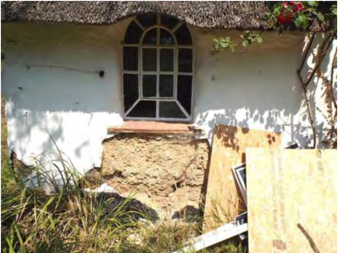
Fig 3.5.8; Bathroom window with decayed wall face & render below
