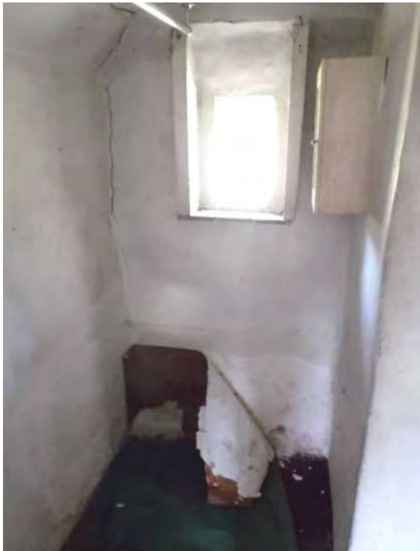
Fig 4.4; Lobby in northwest corner showing crack
