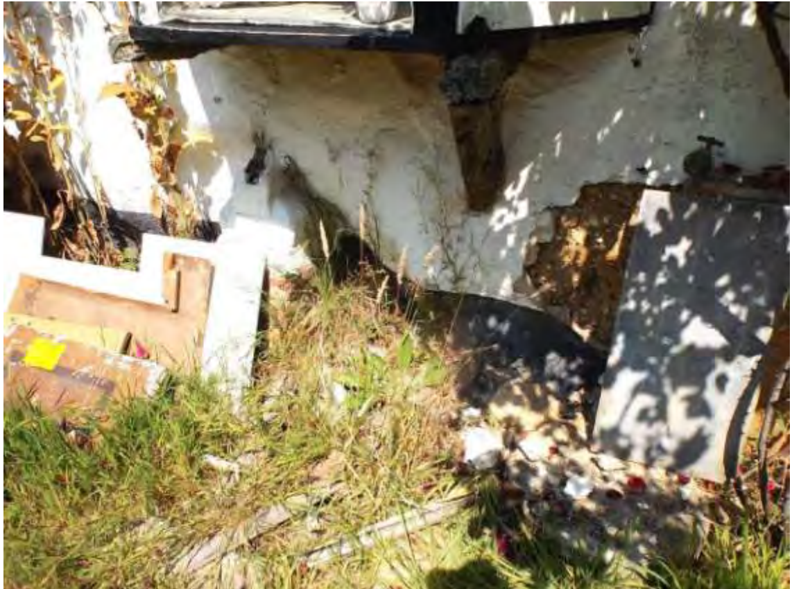
Fig 3.4.16; Rendered wall erosion on south wall
