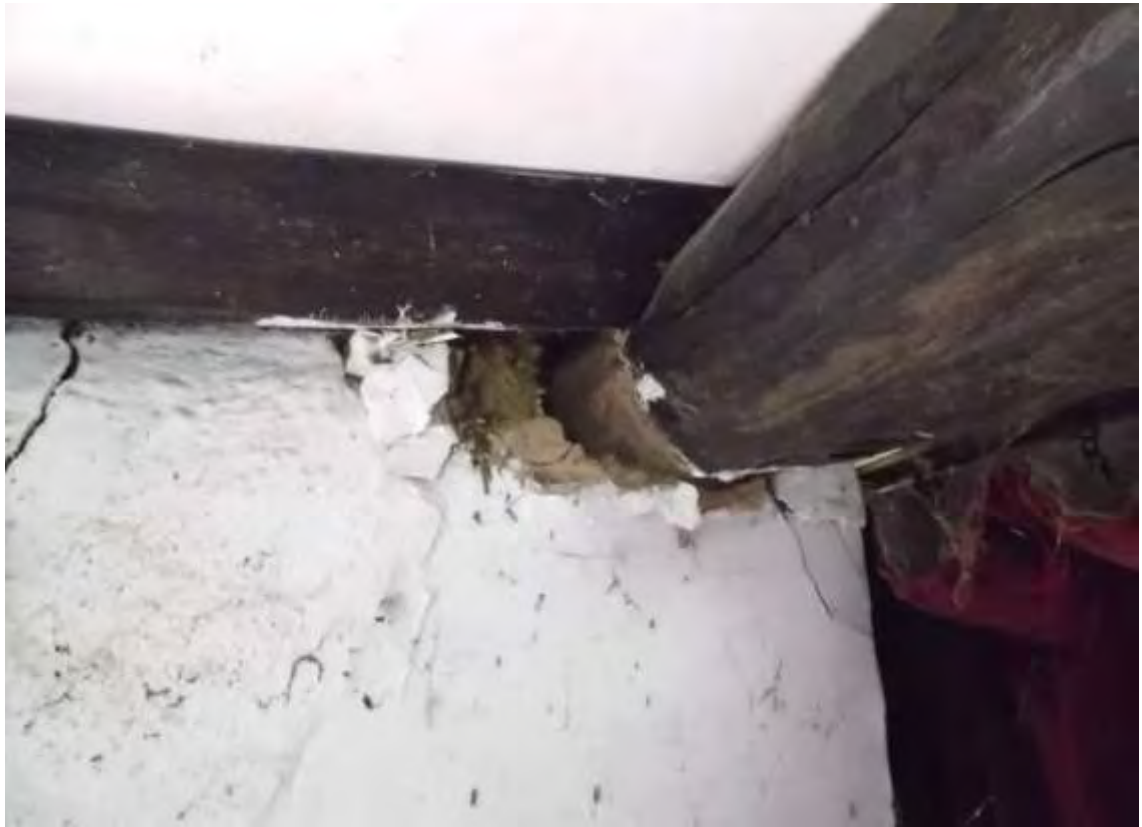
Fig 4.2.12; Displacement of west beam end into south wall
