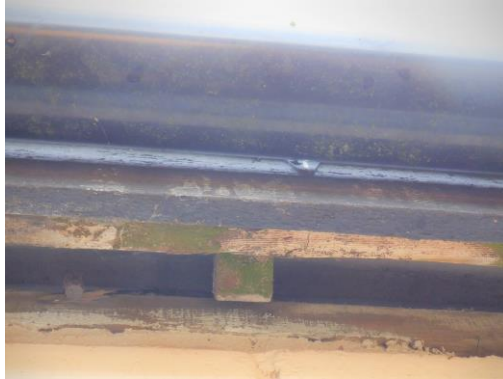
FIGURE 10: SHOWING THE OPEN GAPS AT THE EAVES.
