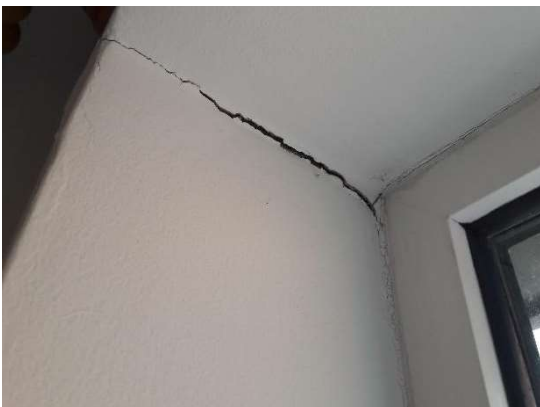
Cracking to Landing Window Head
