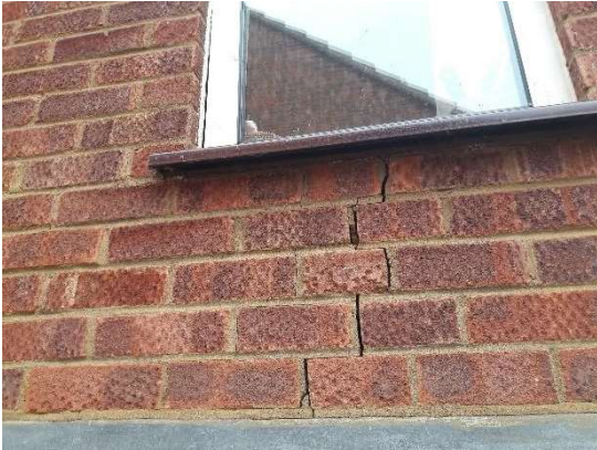
Cracking Below Landing Window
