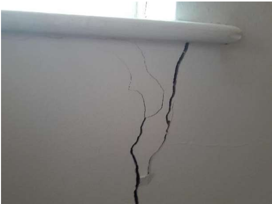
Cracking Below Landing Window
