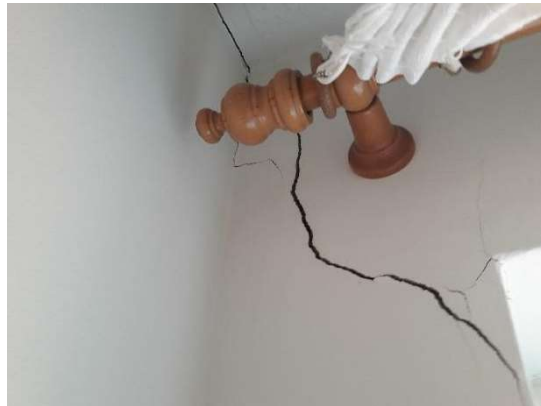
Cracking Above Landing Window
