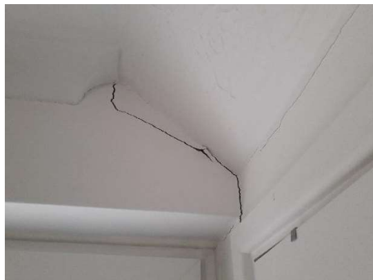
Cracking Above External Door
