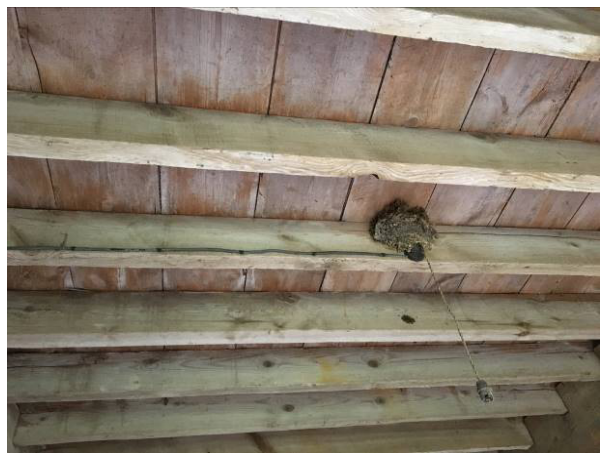
Swallow nest on ceiling joist.
