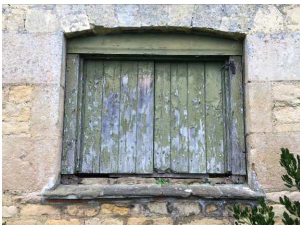
Window to first floor with gaps
