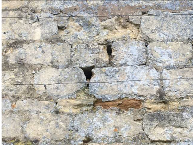
Significant cavities – front of building
