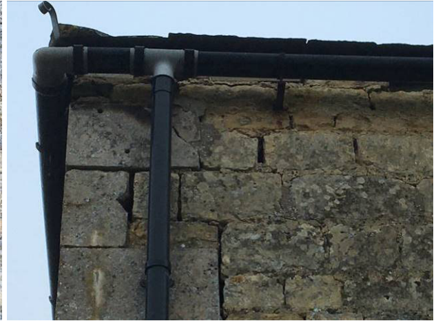
Significant cavities – south west corner.
