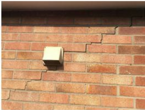
Stepped Crack to Side Wall
