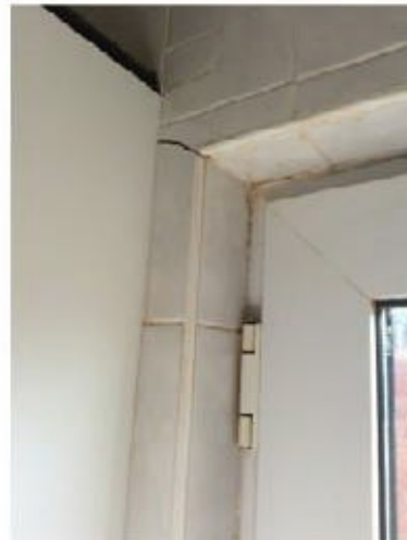
Cracked Tiling Above Rear Door
