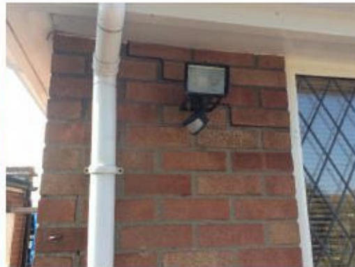
Stepped Crack to Rear Wall
