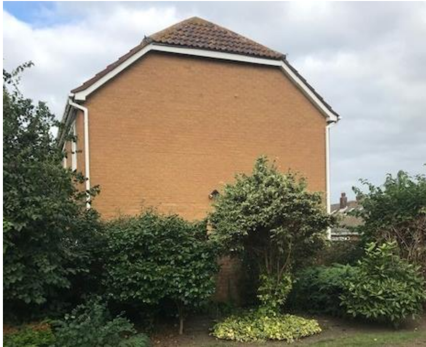
View of flank wall of 1 Moat Croft facing east towards application site
