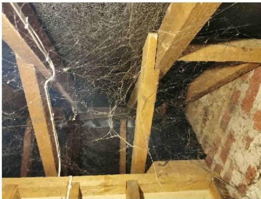
Image 5. Cobwebs in roof space
