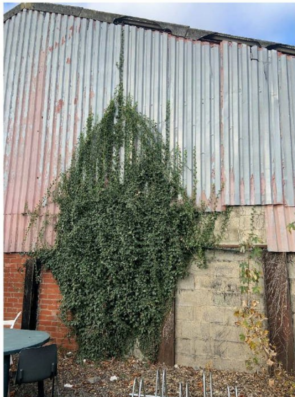
Photograph 13: Ivy on the southern elevation of Billy's Barn
