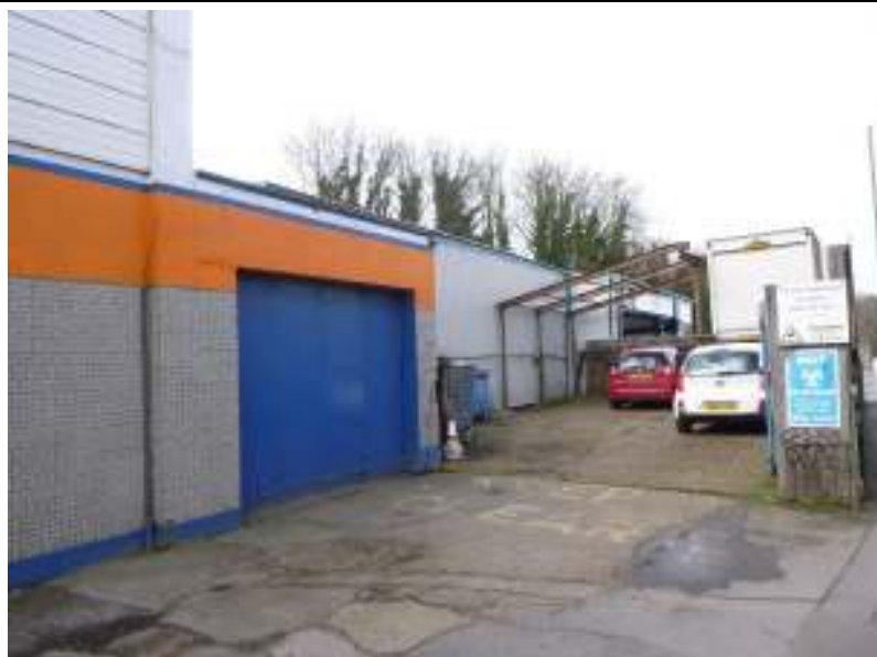
View to the west showing north western forecourt area containing steel remains of former structure.
