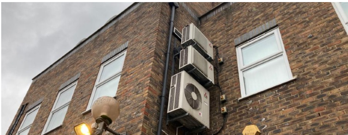
Fig. 6 - Rear Elevation air conditioning units
