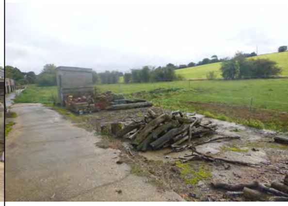
Photo 6 - Wood and construction supplies south of Barn B
