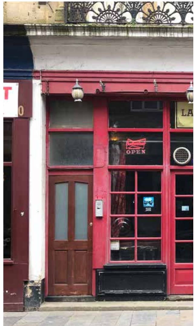
Connection between the two existing shop fronts and existing steps to the threshold of No. 132
