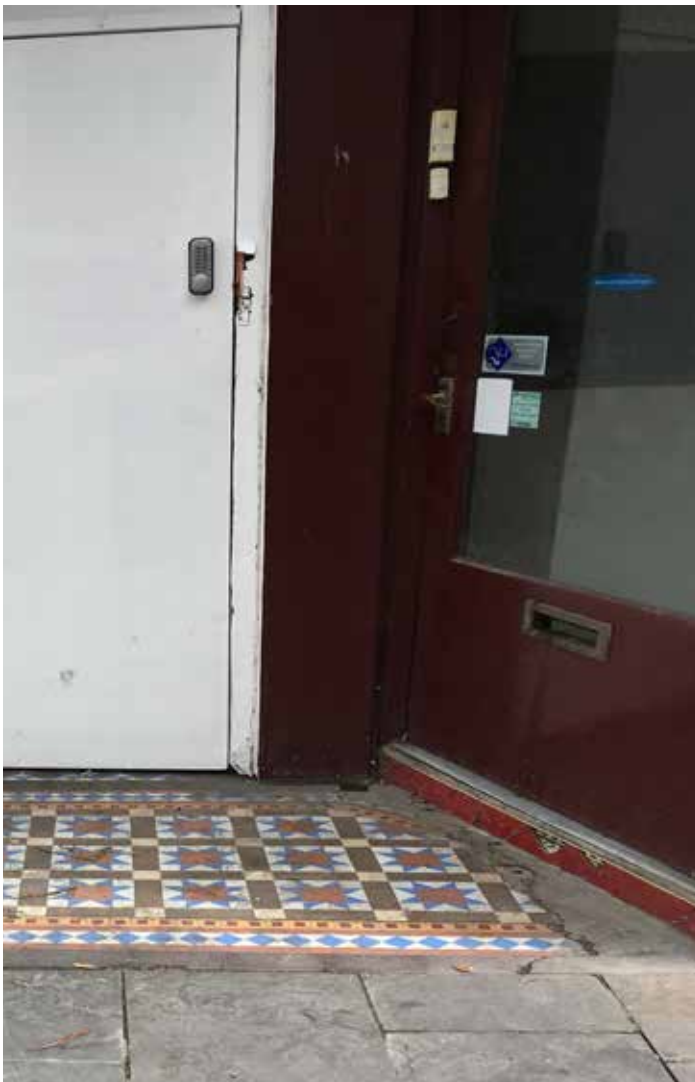
Existing entrance to 'The Stage Door' and condition of geometric patterned tiled Flooring.
