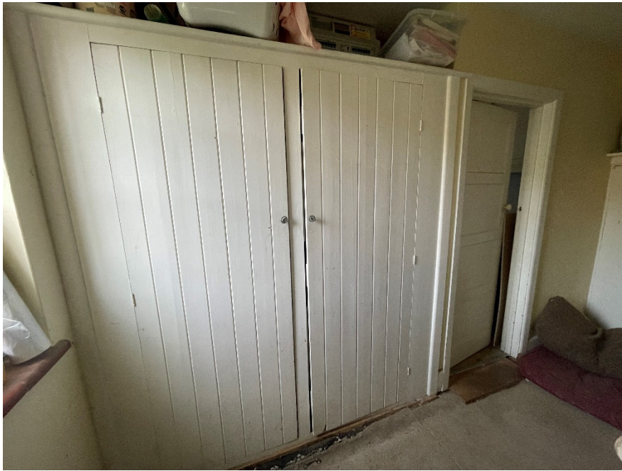
Point No 1. Current cupboards in entrance hall removed to create new kitchen entrance
