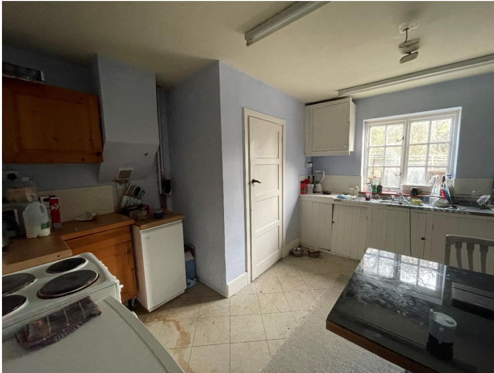
Point No 3. Current kitchen larder to be removed. Also shows redundant chimney breast to be removed.
