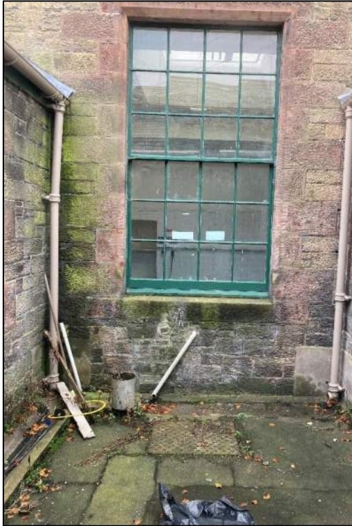
Plate 12: Service yard to east of B26 showing sink drainage under sash window (proposed for removal)
