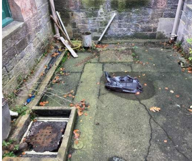
Plate 13: Service yard showing concrete finish and the extant grease trap to bottom LHS of frame
