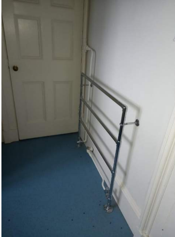
Heated rail to be removed
