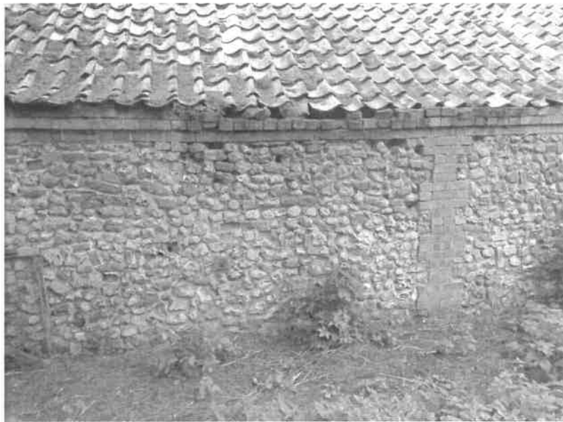
P9: West wing: Lateral movement and localised damage to eaves level corbelled masonry
