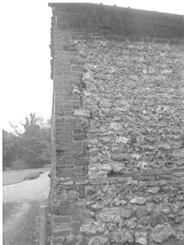
P10: West Wing: Washout of masonry and debonded historical cement fillet repairs at junction between single and two storey sections of west elevation
