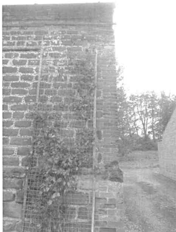
P8: West Wing: Vertical cracking to north east corner of two storey barn
