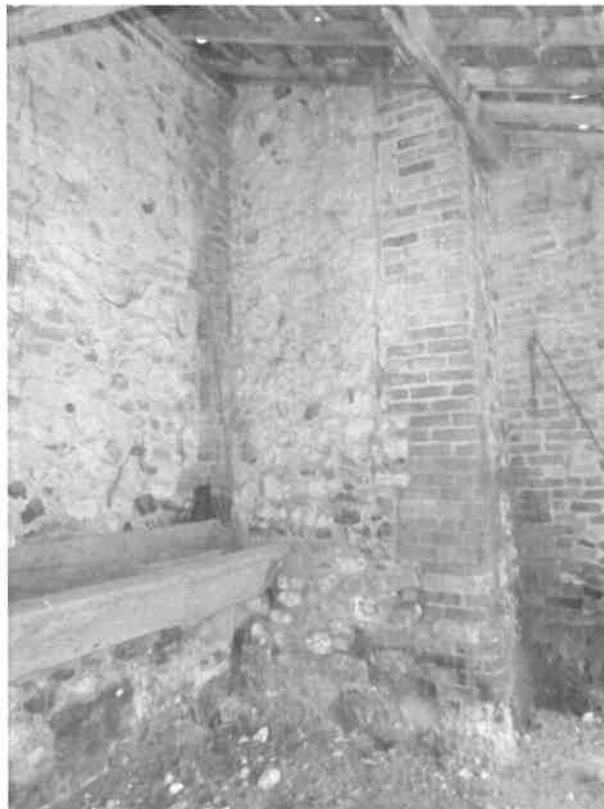
P12: West Wing: Vertically cracking within flintwork panels and corner quoins within lean-to section
