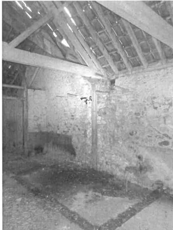
P3: Southern single storey barn: Leakage through roof at bottom of rotten valley member causing localised washout of mortar to walls
