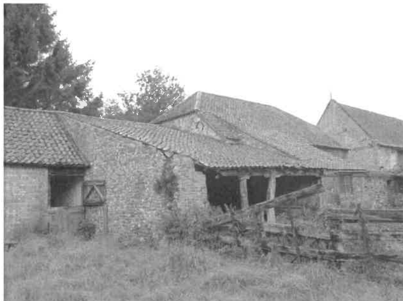
P6: West Wing: Rotten eaves beam to central lean-to section with localised cracking / voiding and vegetation growth
