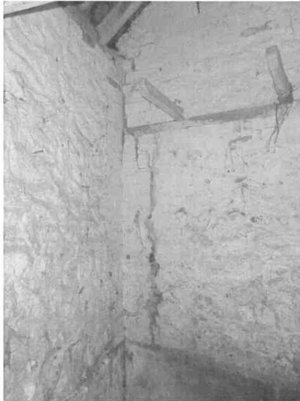
P4: Southern single storey barn: Lateral movement of between 30mm to 40mm evident to internal gable masonry at junction within west wing
