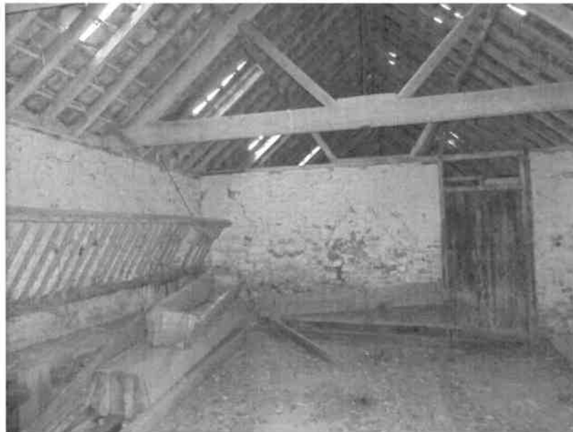
P2: Southern single storey barn: Typical cracking due to lateral movement is evident to a number of cross walls at junction with perimeter walls
