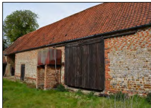
Figure 15 – Western elevation of Main Barn 4 Complex showing a wooden access door where gaps were present
