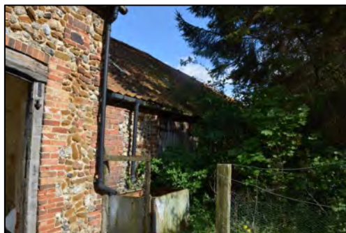
Figure 18 – Western elevation of Barn G, showing overgrown bushes covering the elevation
