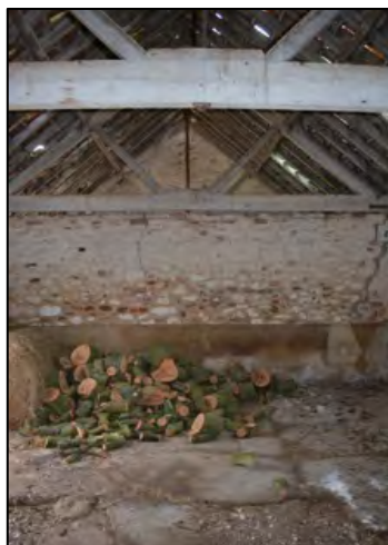
Figure 26 – Internal view of Barn 4 Complex (section F), showing its poor state of repair
