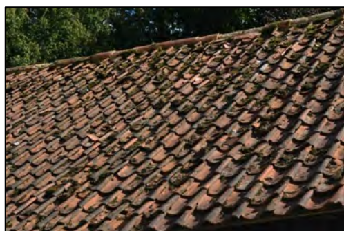
Figure 45 – Lightly mossed western elevation pantile roof, with gaps between the pantiles
