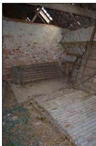
Figure 25 – Internal view of Barn 4 Complex (section E), showing general use and the poor state of repair
