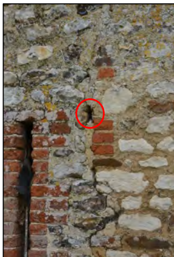
Figure 38 – Large clear cavity on the external northern wall
