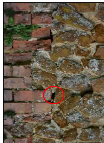
Figure 37 – Lower cavity where a common pipistrelle was noted roosting on the south-western elevation of Barn E
