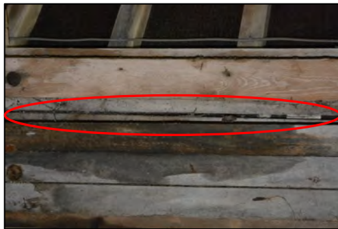
Figure 34 – Feature between the lintel and door frame that a barbastele was found on the eastern elevation of Barn C
