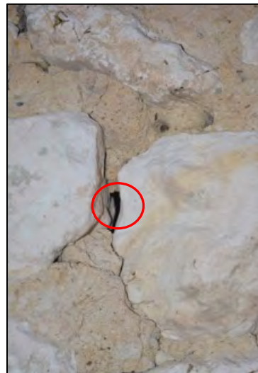
Figure 35 – Internal cavity in Barn E – made smooth by bat activity
