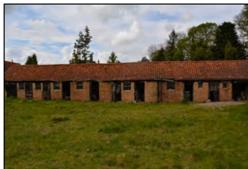
Figure 19 – Southern view of Main Barn 4 Complex (section J), showing the damaged doors and windows
