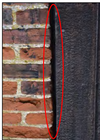
Figure 36 – Feature between the door frame and wall where a common pipistrelle was noted roosting on the west elevation of Barn C – external
