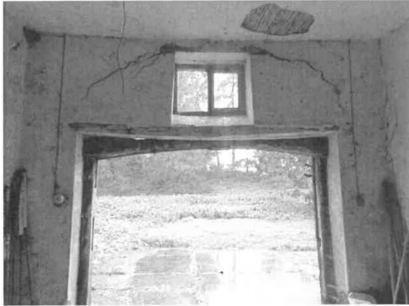
P13: West Wing: Diagonal cracking above arched timber lintel within workshop
