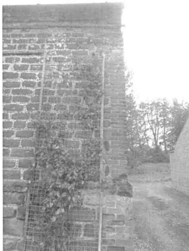
P8: West Wing: Vertical cracking to north east corner of two storey barn
