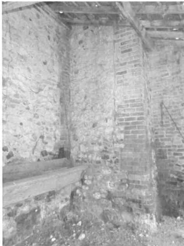
P12: West Wing: Vertically cracking within flintwork panels and corner quoins within lean-to section
