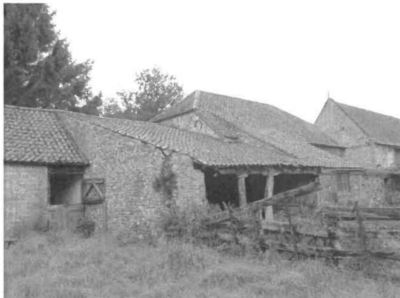
P6: West Wing: Rotten eaves beam to central lean-to section with localised cracking / voiding and vegetation growth
