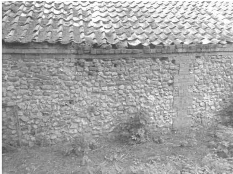
P9: West wing: Lateral movement and localised damage to eaves level corbelled masonry
