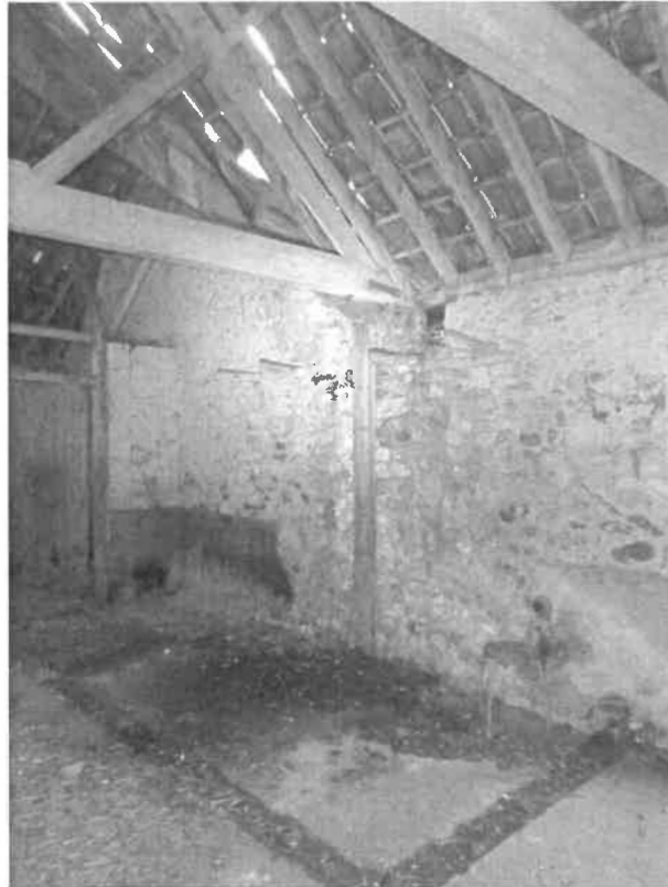
P3: Southern single storey barn: Leakage through roof at bottom of rotten valley member causing localised washout of mortar to walls
