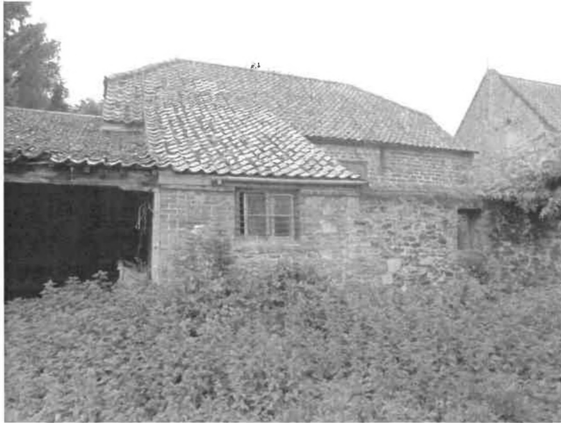
P7: West Wing: Cracking and weathered masonry to courtyard facing lean-to
