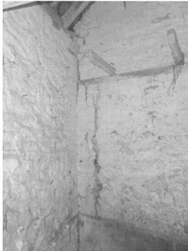
P4: Southern single storey barn: Lateral movement of between 30mm to 40mm evident to internal gable masonry at junction within west wing
