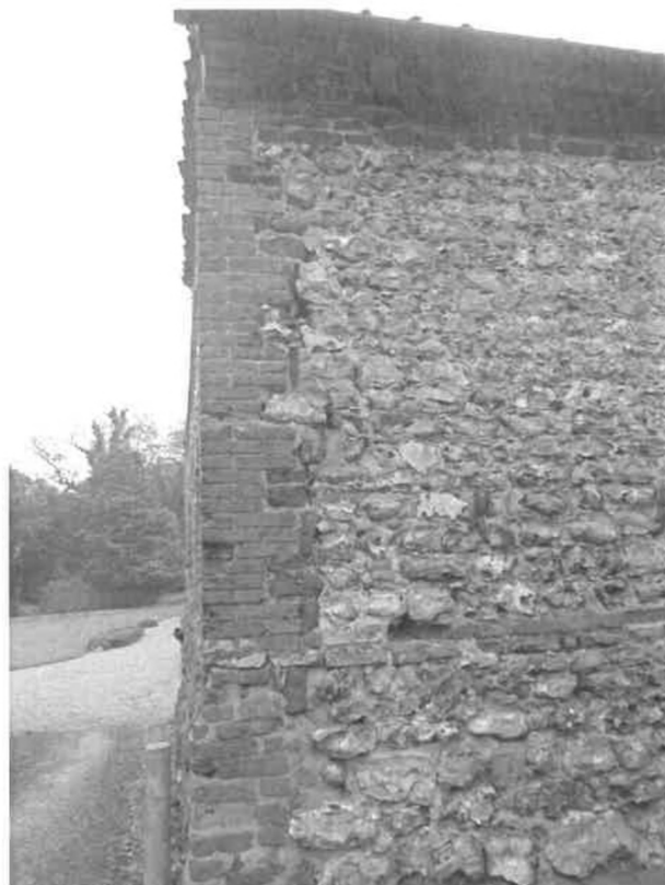
P10: West Wing: Washout of masonry and debonded historical cement fillet repairs at junction between single and two storey sections of west elevation
