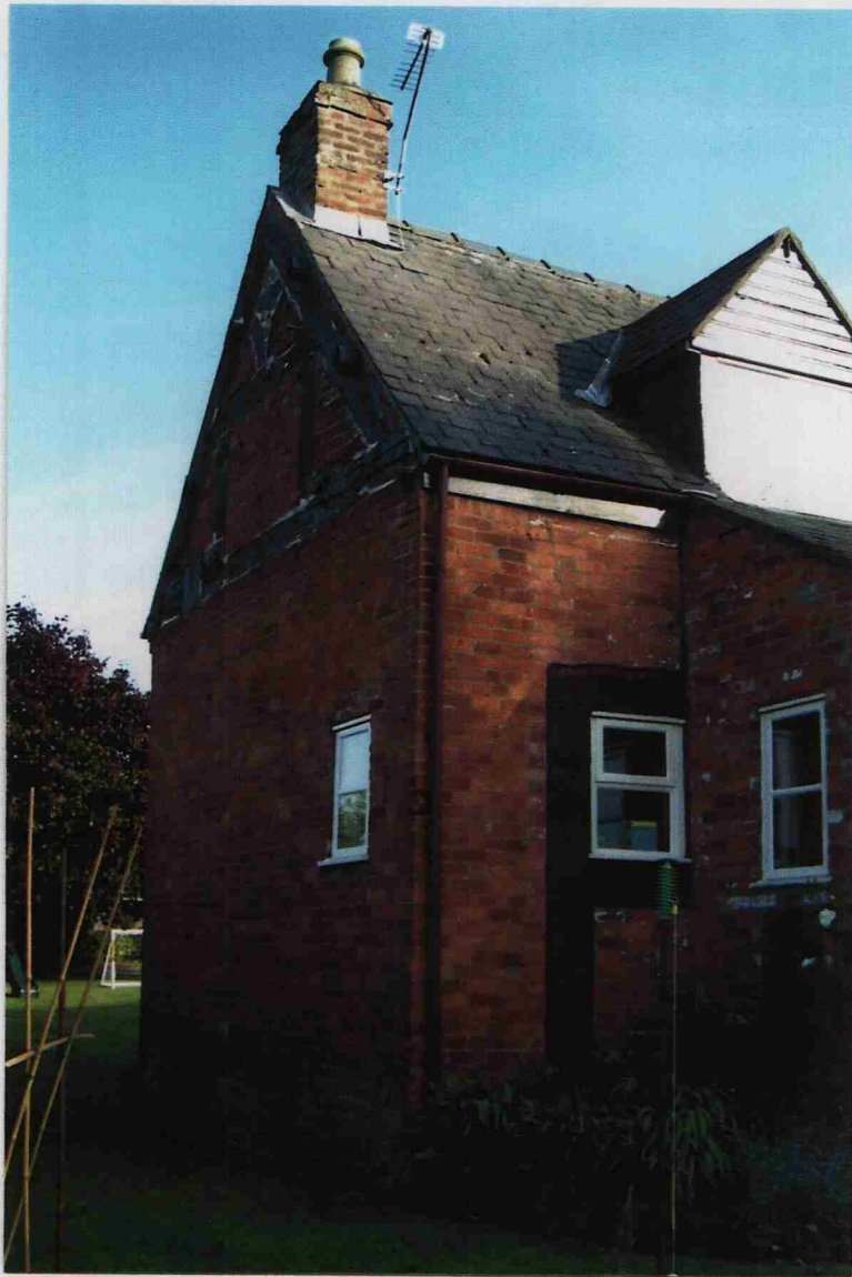
PHOTOGRAPH 2 - GENERAL VIEW OF THE END GABLE WALL OF THE ORIGINAL PART OF THE COTTAGE. IN THE GABLE IS ONLY PART OF THE ORIGINAL TIMBER FRAMED BUILDING WHICH IS EXPOSED EXTERNALLY ALONG WITH THE SMALL SECTION ON THE REAR WALL WHICH CAN ALSO BE SEEN IN THIS PHOTO.
