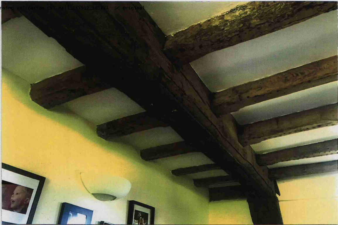
PHOTOGRAPH 6 - DETAIL OF THE CEILING STRUCTURE WITHIN THE CORE OF THE ORIGINAL HOUSE.
