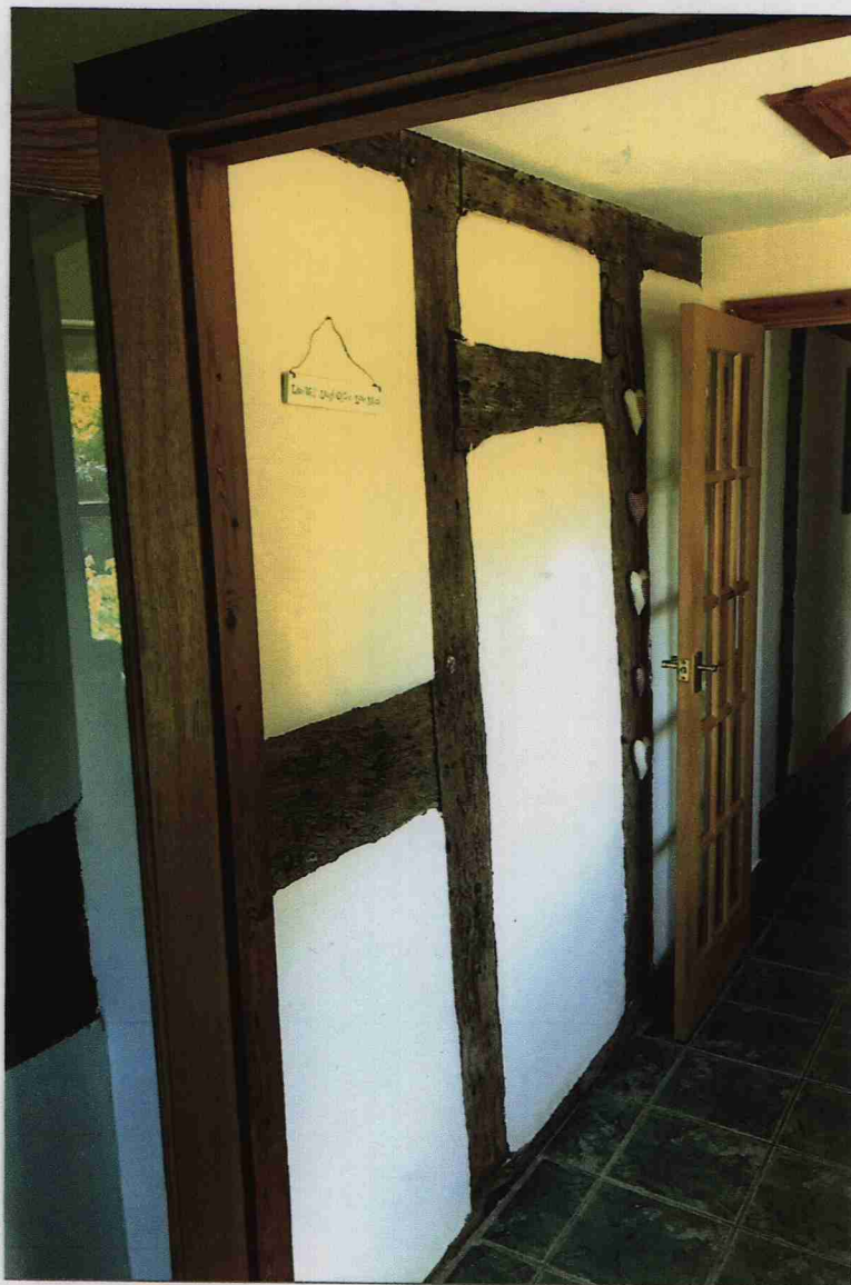
PHOTOGRAPH 5 - DETAIL OF THE TIMBER FRAMING TO THE REAR WALL WHICH IS PRESERVED INTERNALLY WITHIN AN OLDER LEAN TO ADDITION.
