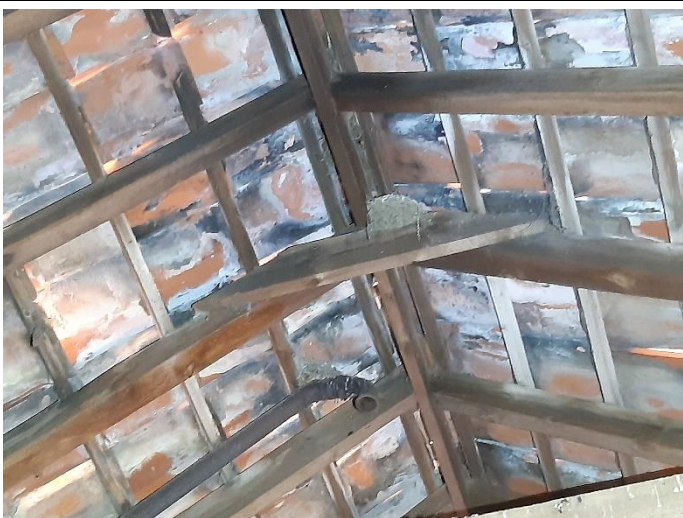
Photo 11 Interior of pantile roof, showing gaps, absence of roofing membrane and swallow nest adjacent to ridge
