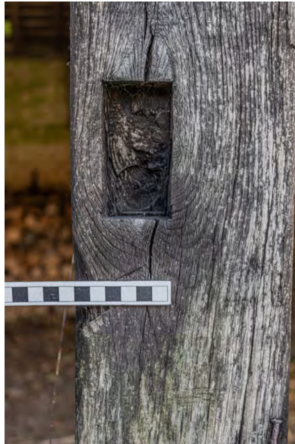
Plate 29 (022): Cart Store, North-West Elevation, detail of slot in the north-west facing side of post from the north-west
