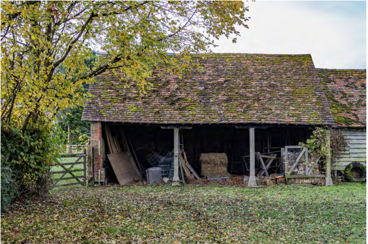
Plate 47 (036): Cart Store, North-East Elevation, general view of the Cart Store from the north-east
