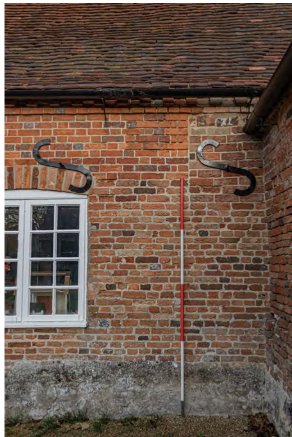
Plate 62 (013): Farmhouse, South-East Elevation, detail of the blocked window in the north-east side, from the south-east
