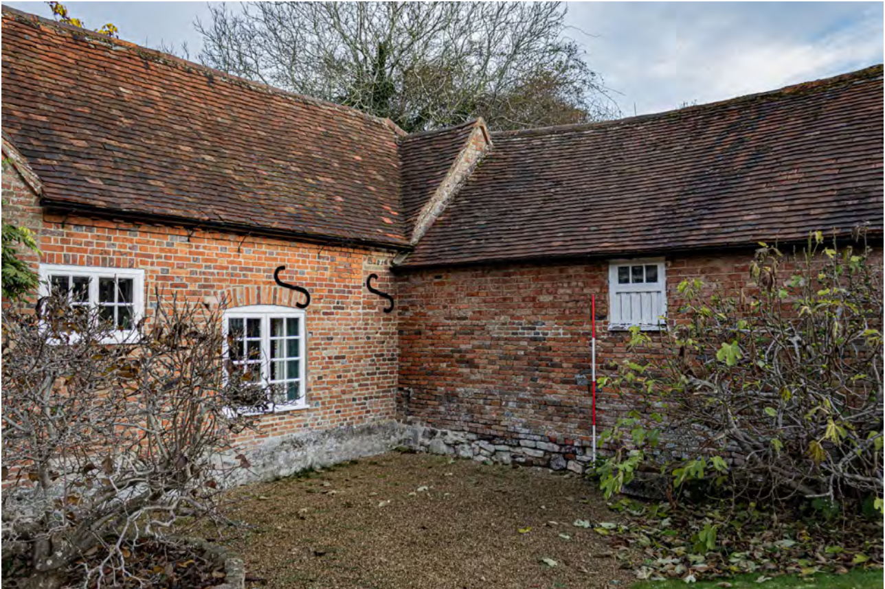
Plate 19 (010): Cow Shed, South-West Elevation, general view of the north-west side, from the SSW
