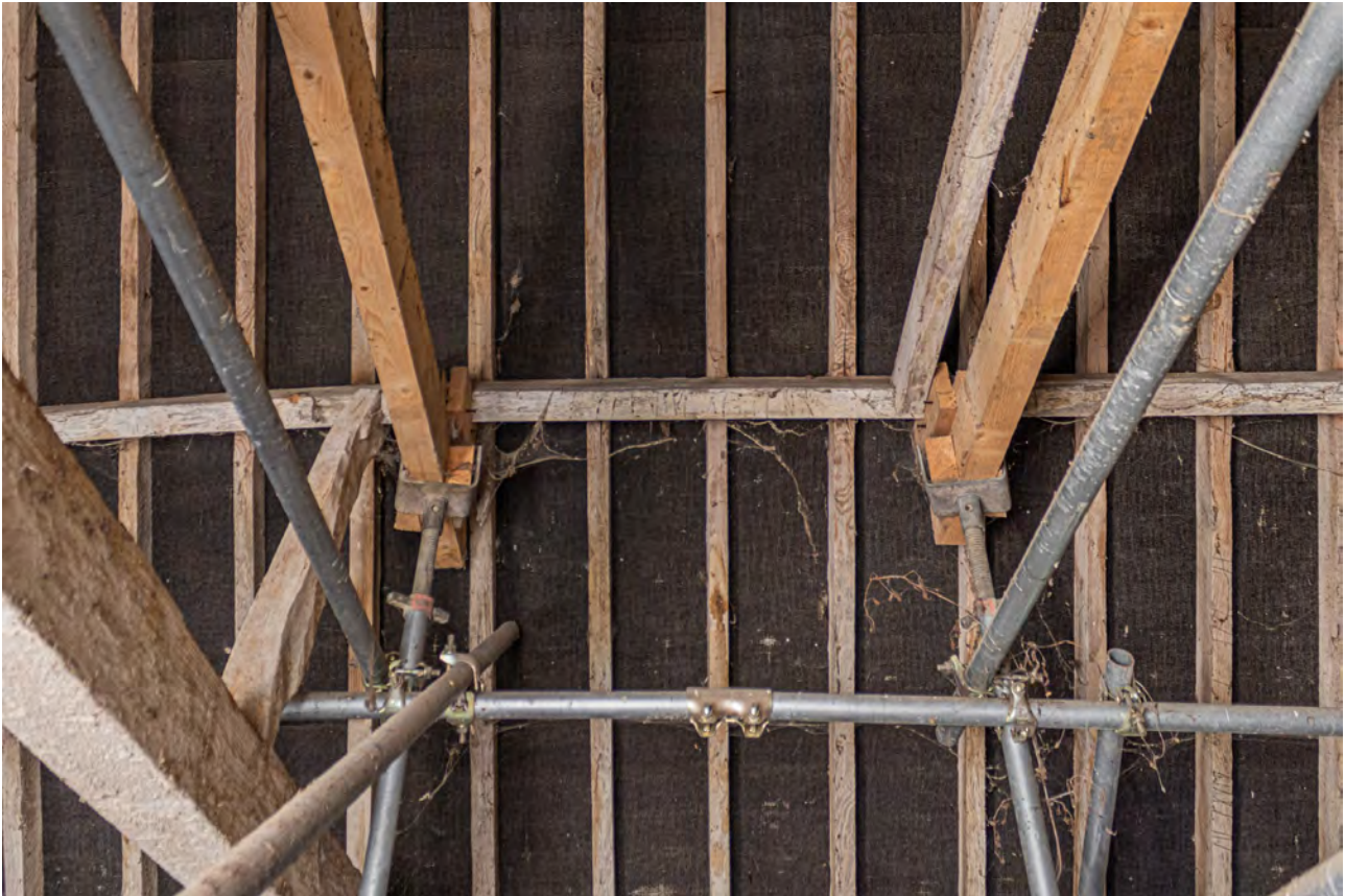
Plate 67 (074): Room 1, detail of the underside of the roof on the north-east side showing the scaffolding poles, from the south-west
