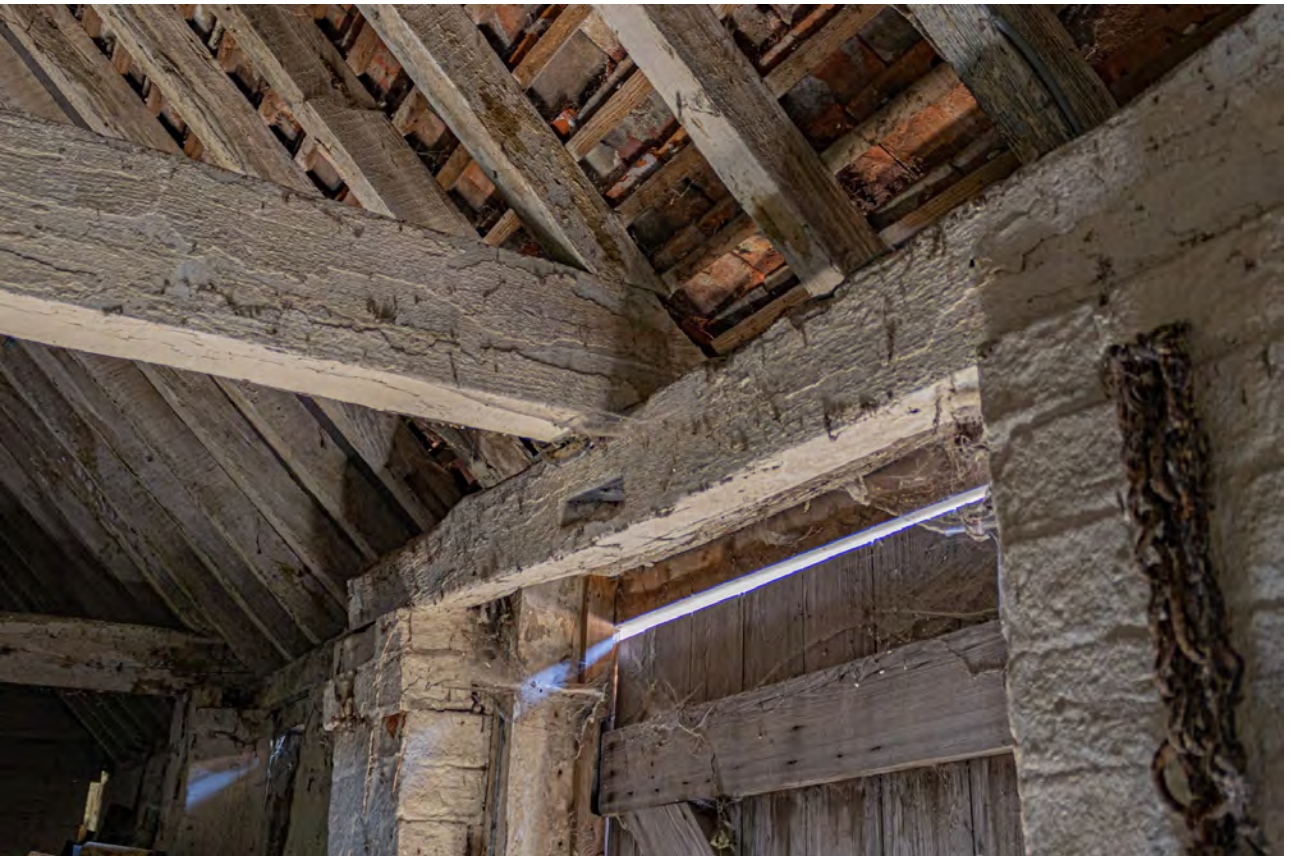
Plate 74 (111): Room 1, detail of timber lintel over the doorway in the south-west elevation, from the north
