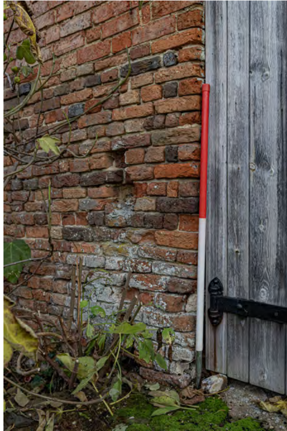
Plate 23 (019): Cow Shed, South-West Elevation, detail of the broken-away brickwork to the north-west side of the doorway, from the south
