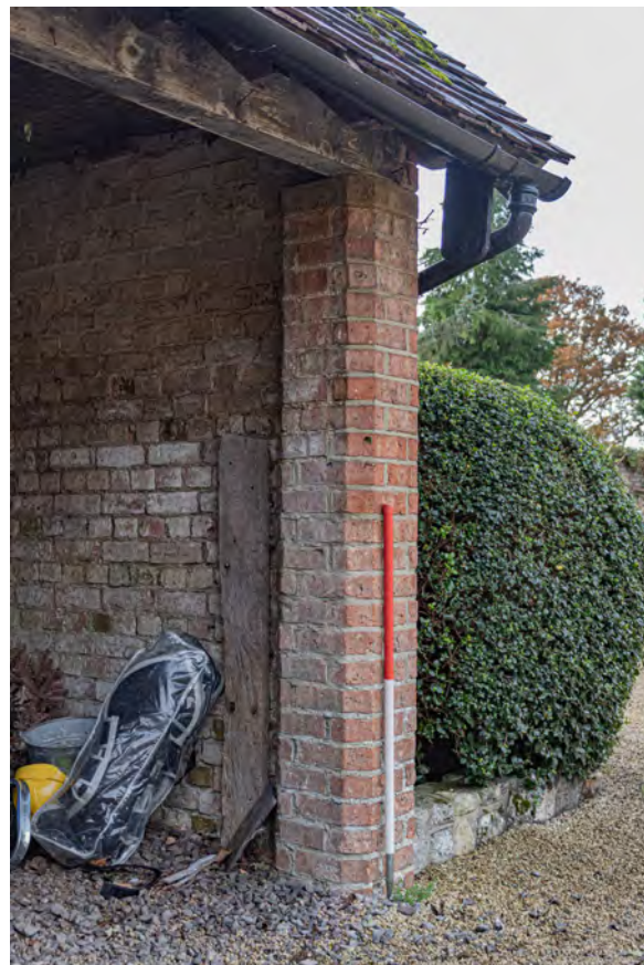
Plate 30 (020): Cart Store, North-West Elevation, detail of chamfered brick post in the south-west side, from the ENE
