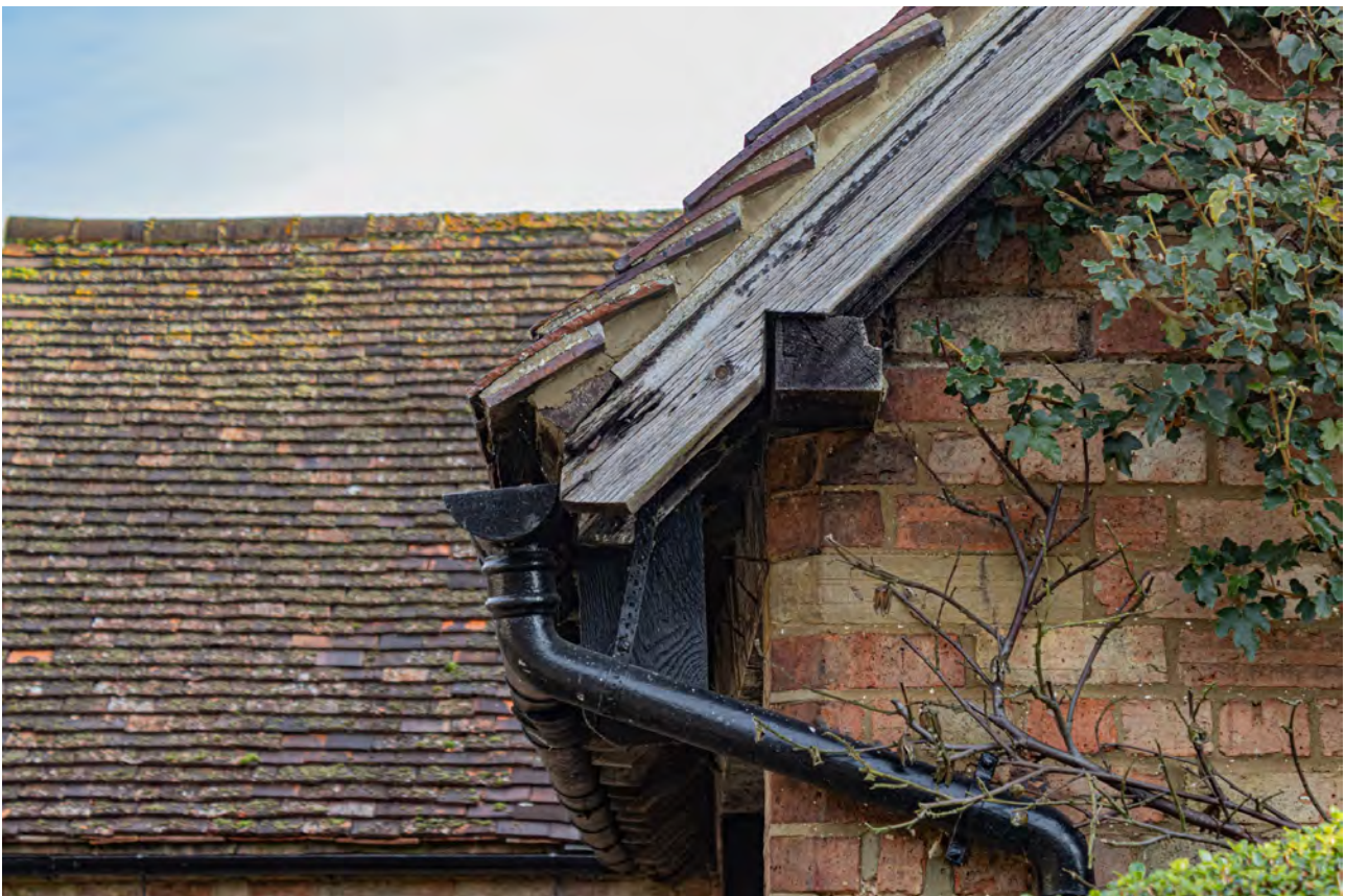
Plate 32 (024): Cart Store, South-West Elevation, detail of the north-west side, from the south-west
