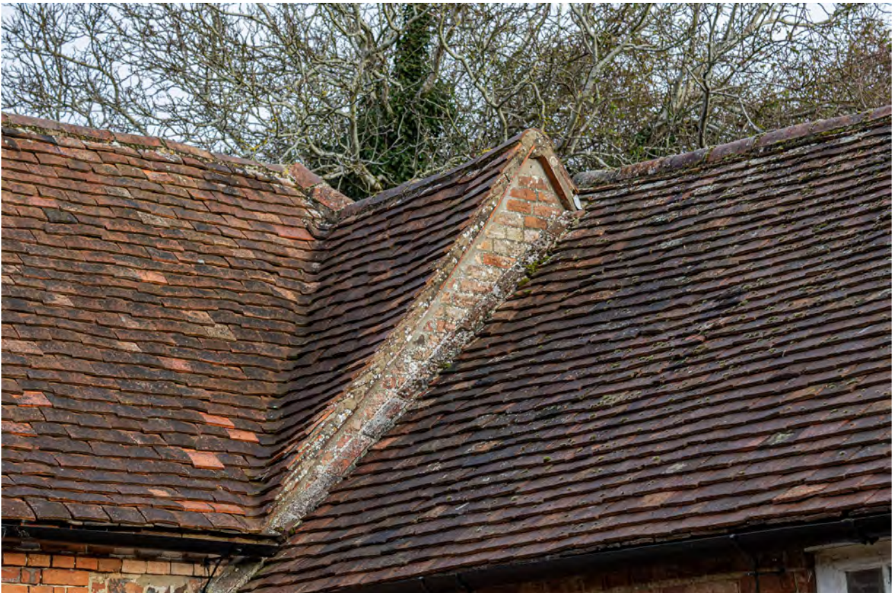
Plate 24 (011): Cow Shed, South-West Elevation, detail of gable of Farmhouse rising above the Cow Shed, from the south
