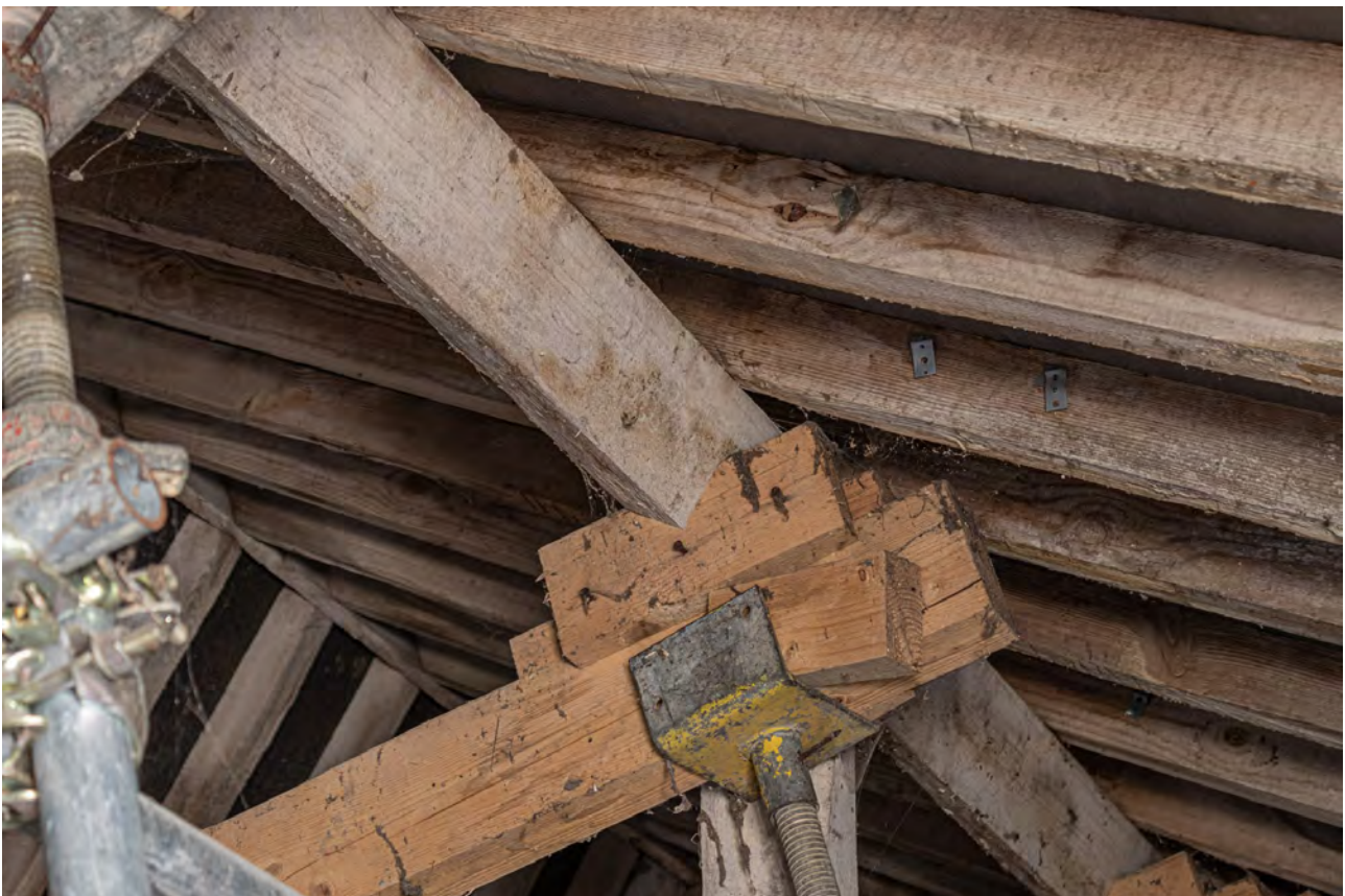
Plate 68 (069): Room 1, detail of supporting scaffolding pole supporting the purlin beams, from the WNW
