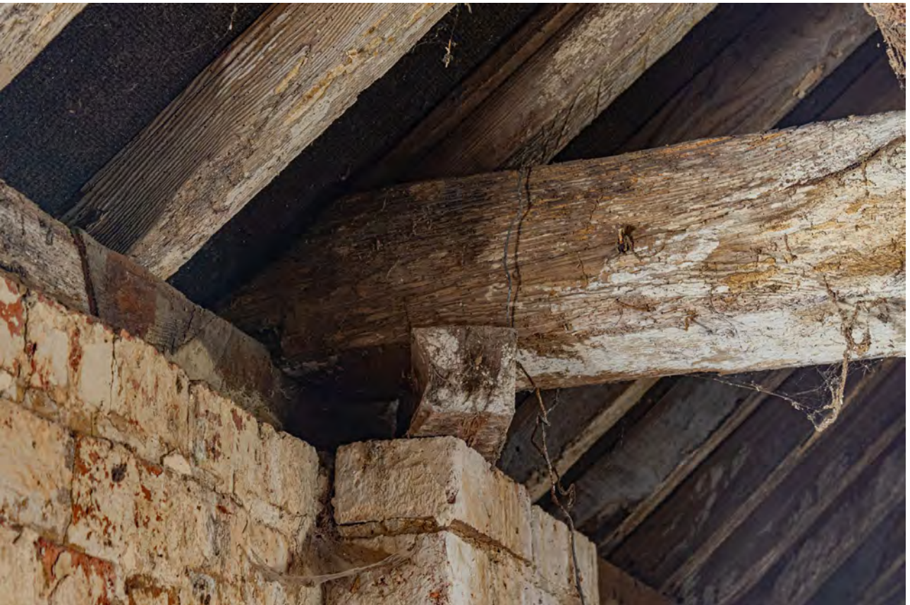
Plate 78 (107): Room 1, detail of tie beam of Truss A resting over wall [27], from the ESE
