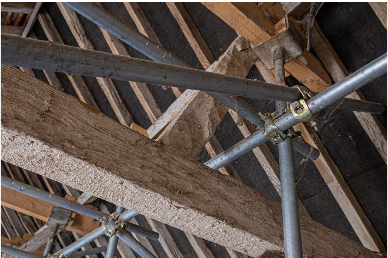
Plate 92 (073): Room 1, detail of south-east facing side of the north-east cross strut of Truss C, from the SSE
