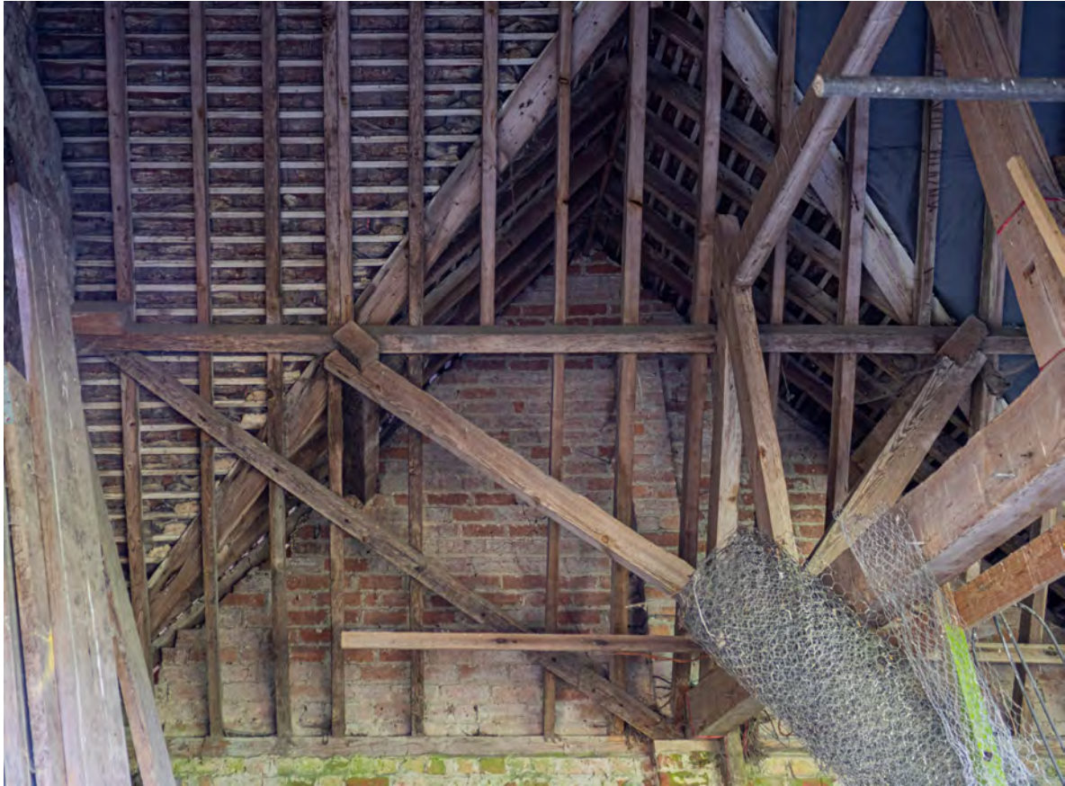
Plate 117 (103): Room 2, general view of the roof structure in the south-east side of the south-east wall, from the north-east
