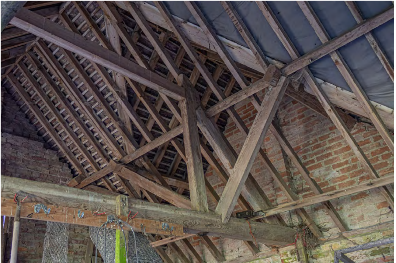
Plate 105 (093): Room 2, detail of Truss F and timber framed roof from the north
