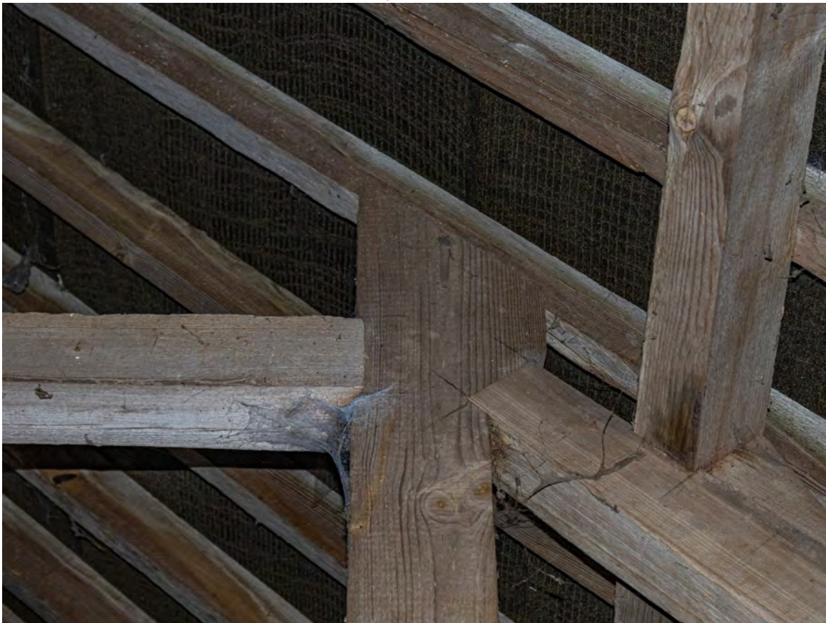
Plate 116 (126): Room 2, detail of top of Queen post connecting to the purlin beam in the north-east side of Truss D, from the south-east
