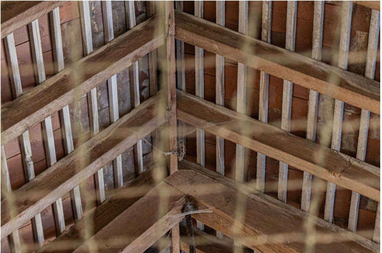
Plate 125 (085): Room 3, detail of tie rod attachment to the upper rafters, from the north-east
