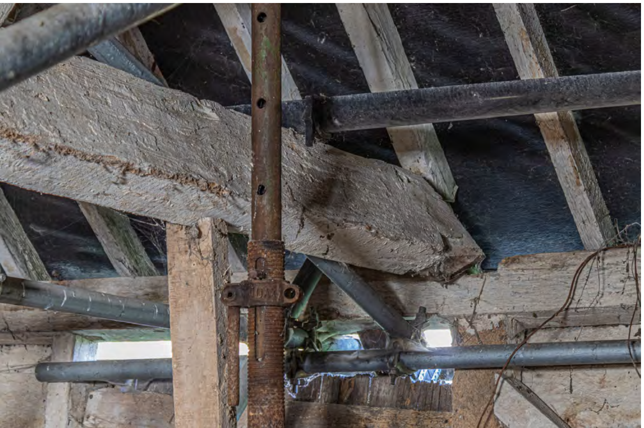
Plate 86 (108): Room 1, detail of tie beam of Truss A in the north-east side, from the south
