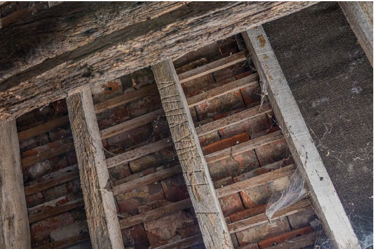
Plate 94 (110): Room 1, detail of marks on the underside of the roof rafter in the south-west side, from the north-east
