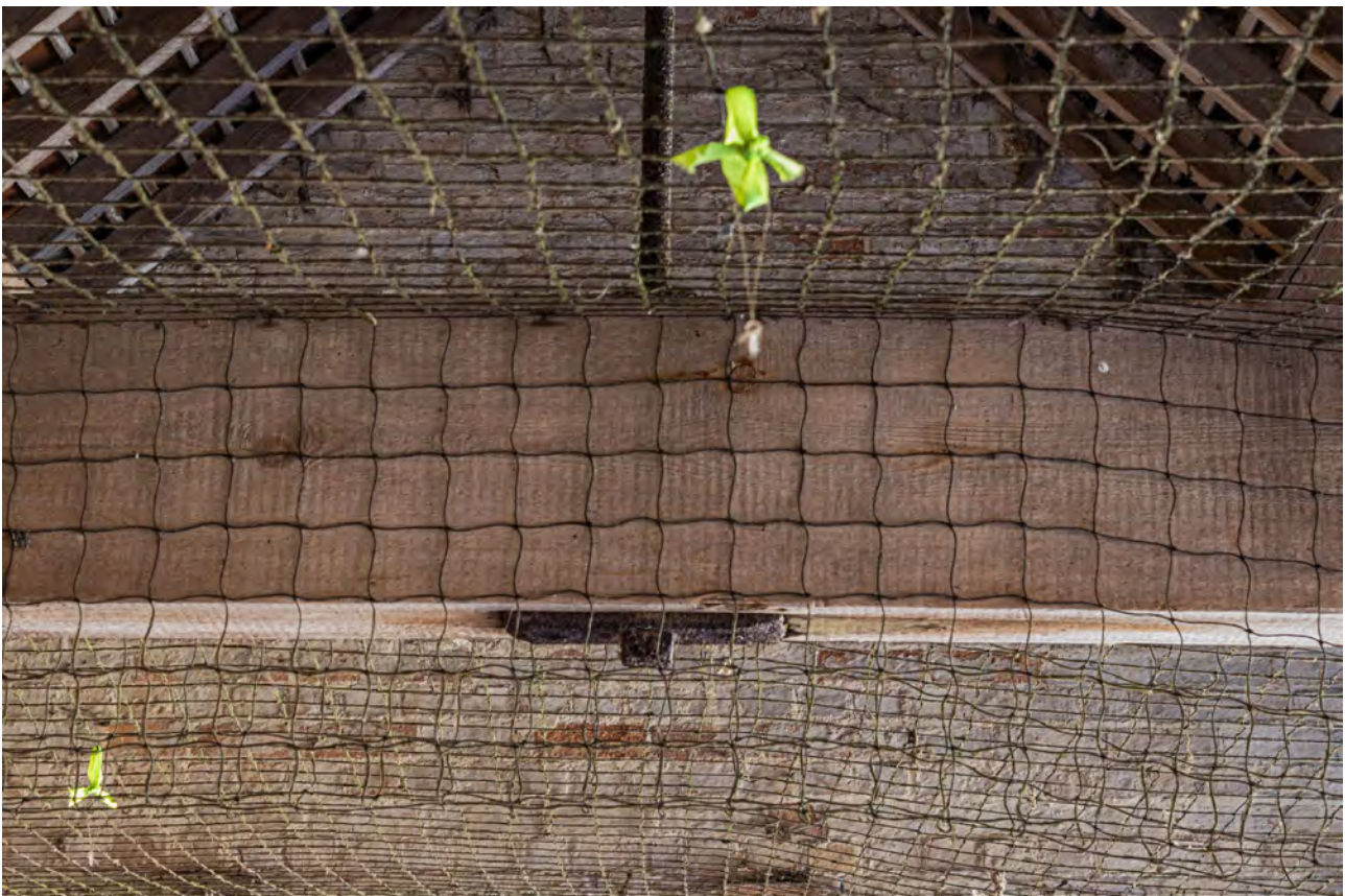
Plate 124 (083): Room 3, detail of base of tie beam showing tie rod attached via a bolt, from the north-east
