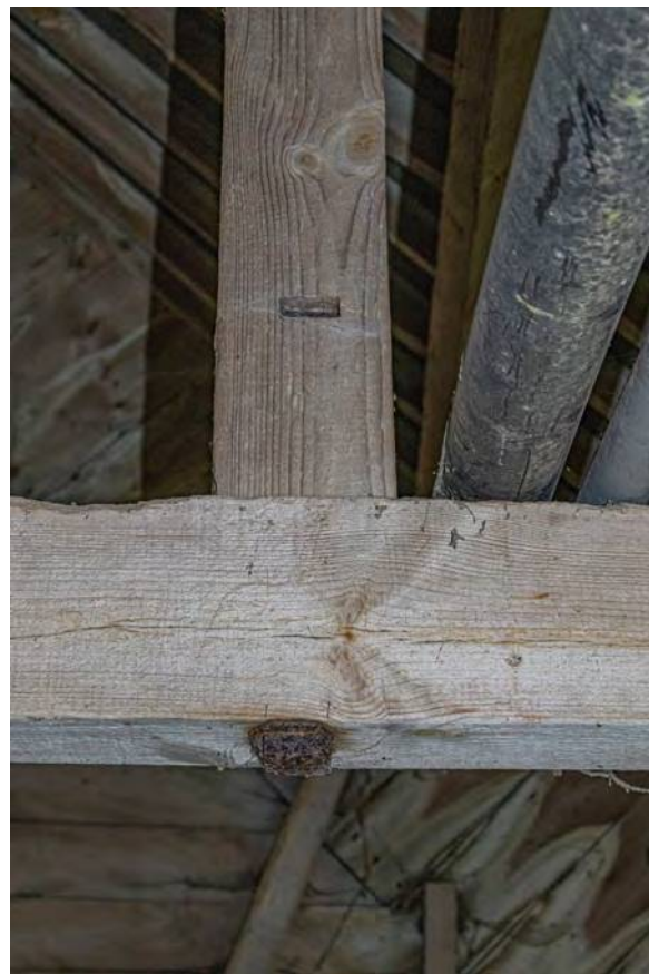
Plate 108 (124): Room 2, detail of north-east Queen post showing slot and tie beam showing bolt to the underside, from the south-east
