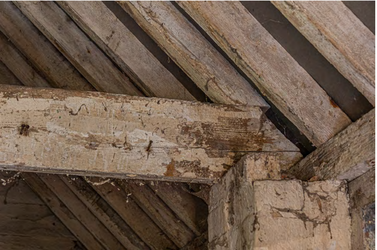
Plate 77 (112/066): Room 1, detail of tie beam of Truss C resting over wall [27], from the north-west
