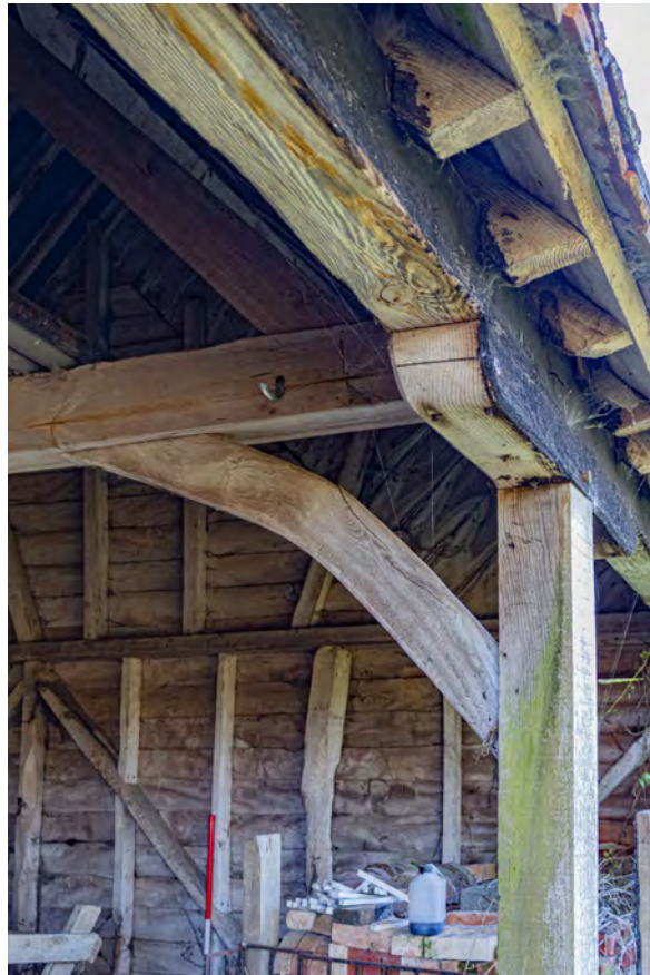
Plate 113 (098): Room 2, detail of top of post [19] in the north-east side and arched brace supporting Truss E, from the ESE
