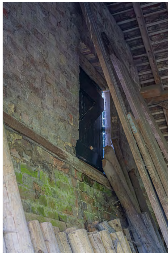
Plate 100 (101): Room 2, detail of loft window [16] in the top of the gable in the south-east wall [33] from the north-east
