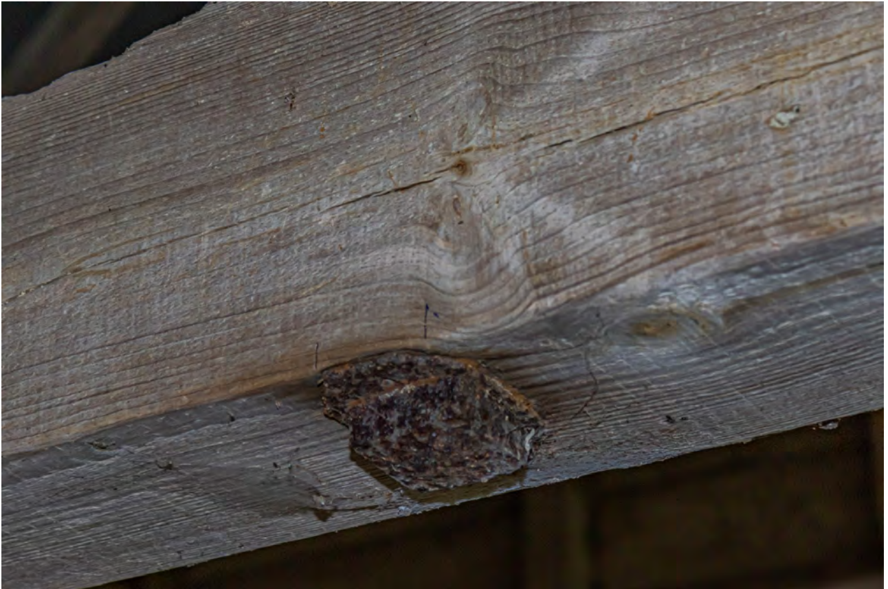
Plate 109 (125): Room 2, close detail of bolt to the underside of the tie beam on the north-east side, from the east
