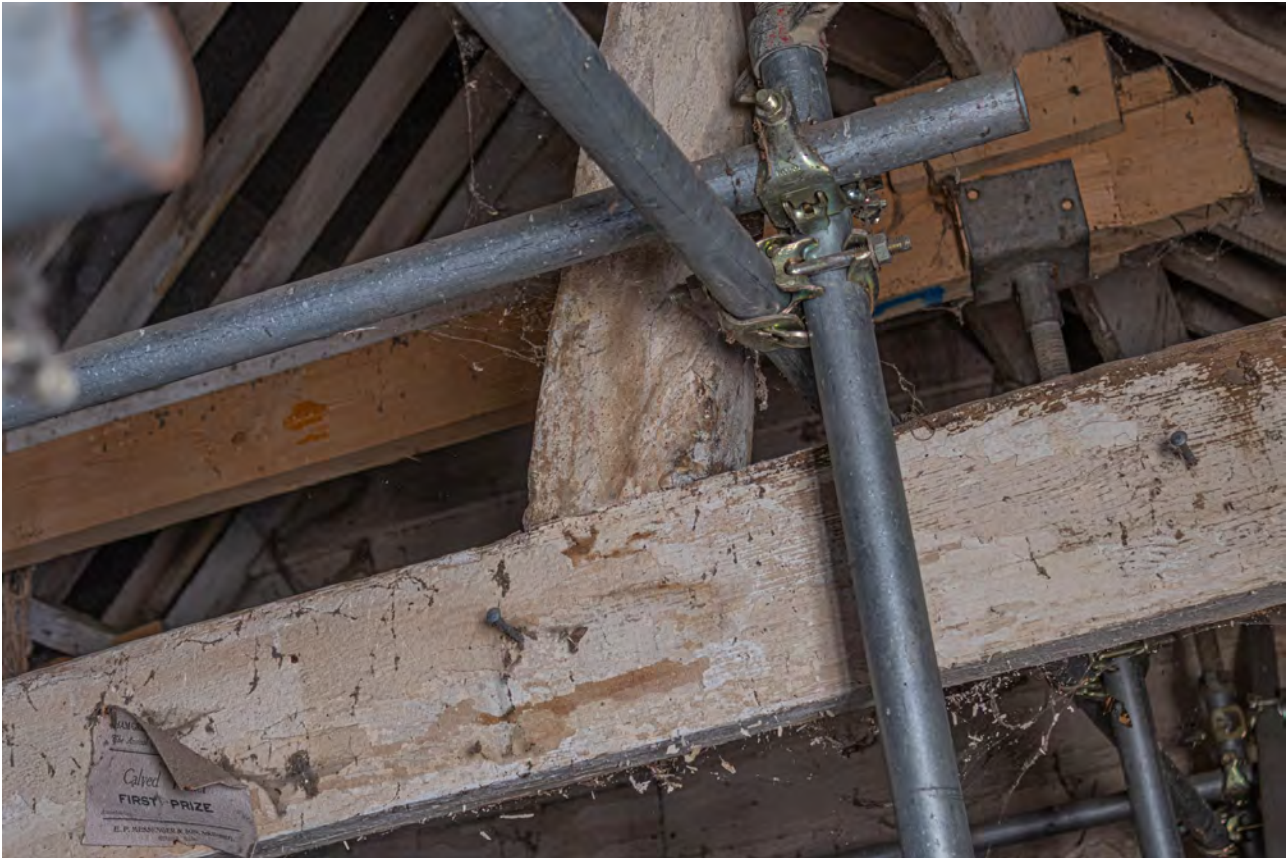
Plate 91 (067): Room 1, detail of the cross strut linking to the tie beam on the south-west side of Truss D, from the WNW
