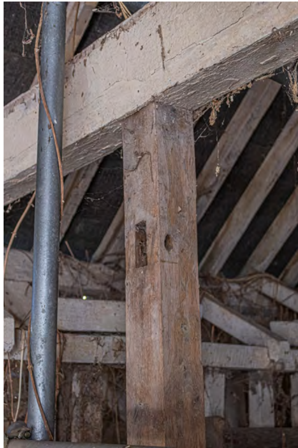
Plate 89 (114): Room 1, detail of post supporting the north-east side of the tie beam of Truss A to the north-east side, from the west
