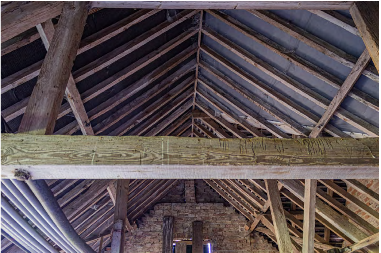
Plate 110 (092): Room 2, detail of north-west facing side of tie beam of Truss E, from the north-west
