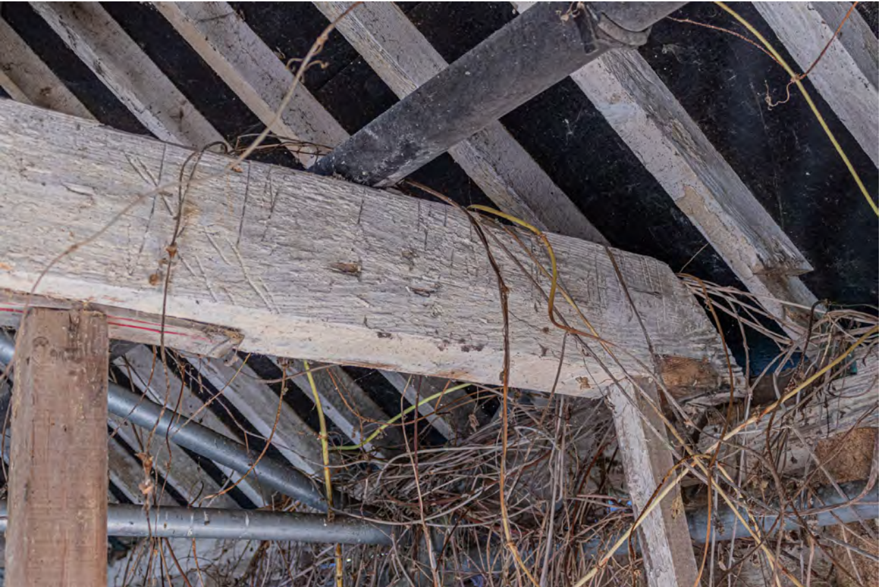
Plate 85 (115): Room 1, detail of tie beam of Truss C in the north-east side, from the south
