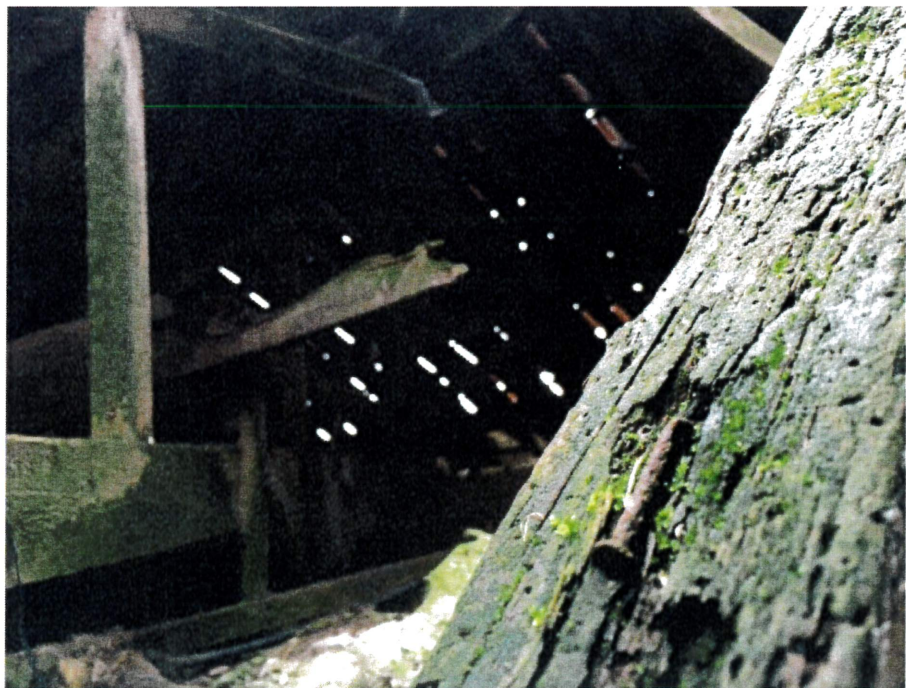
Condition Of Timber Elements Western Barn Were Roof Covering Collapsed
