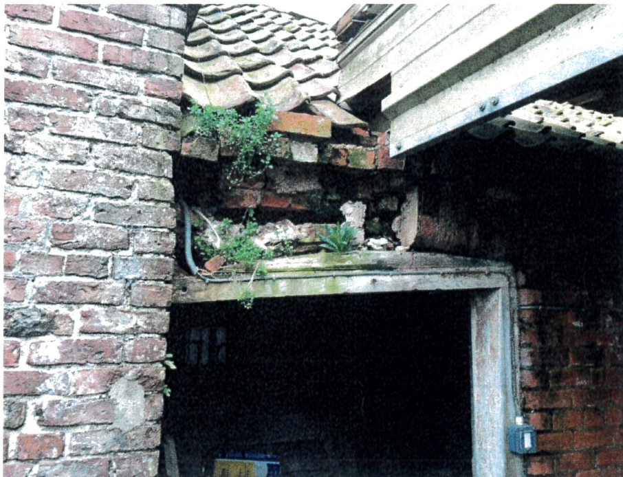
Failed Arch Above Door– North Elevation
