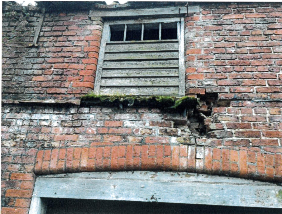
Dislodged Brickwork In Wall Panel– North Elevation
