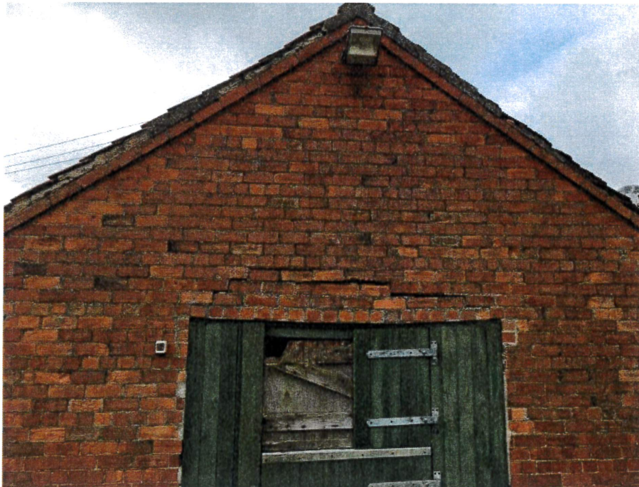
Failed Lintel Above Door – East Elevation
