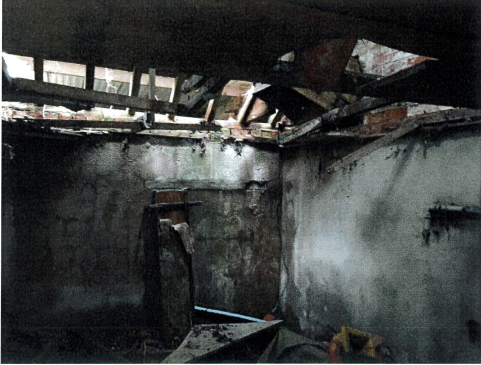
Roof Covering Collapsed - Western Barn
