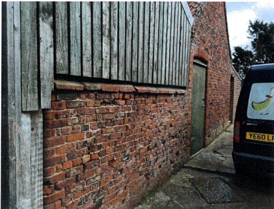
Weathered brickwork – South Elevation
