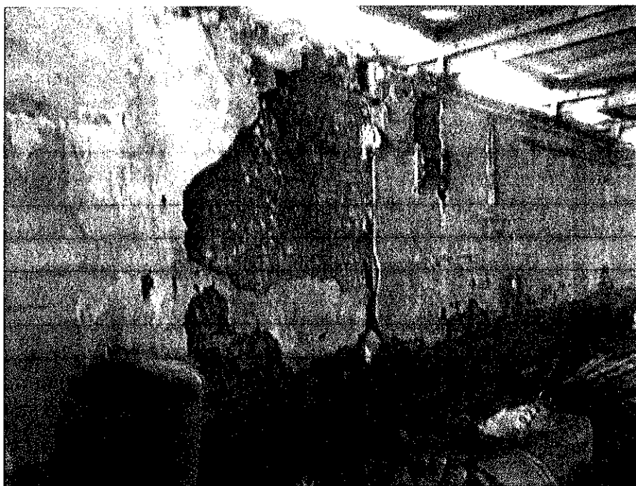
Plate 8. Example of missing render.
