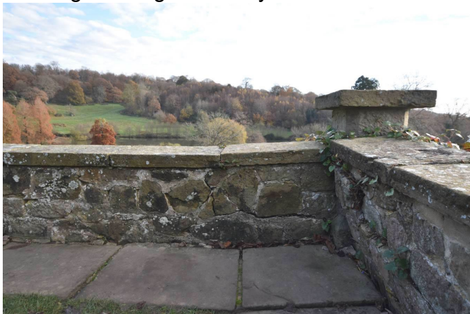
Settlement of terrace wall (photo courtesy of Adrian Cox Associates, Nov 2021)
