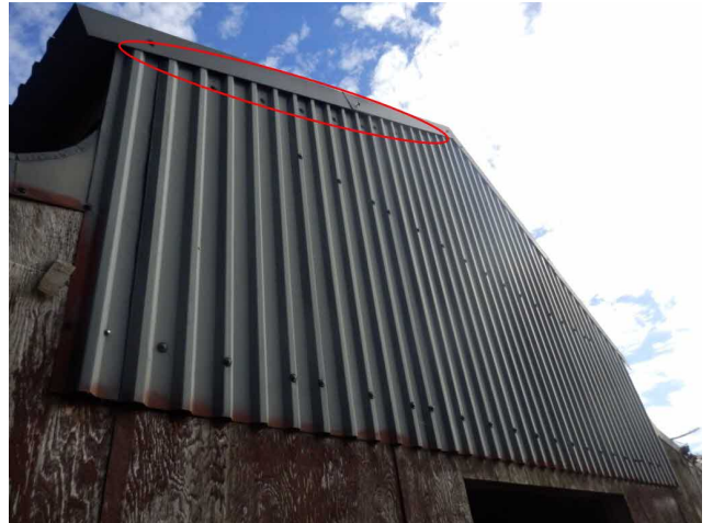
Photo 3. Gap under roof overlap
