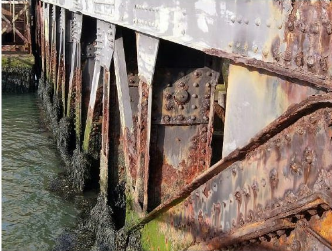
Figure 7 Corrosion has affected many of the steel elements including the linkspan
