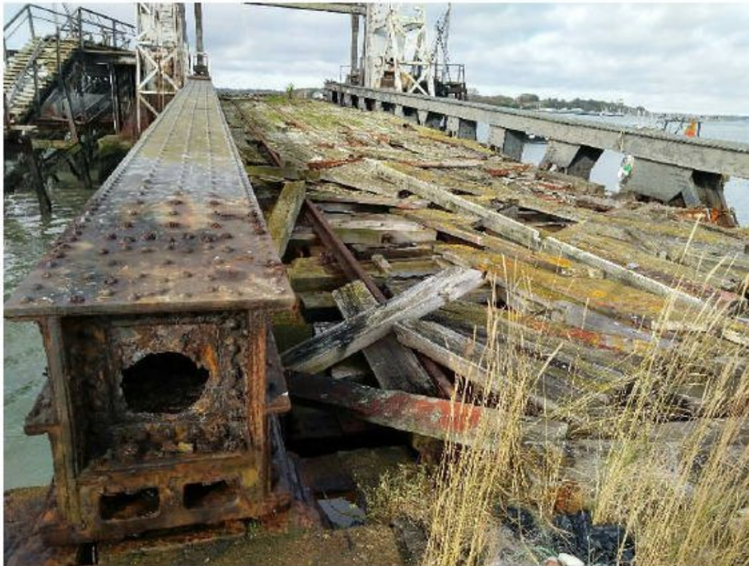
Figure 8 Much of the timber decking is in a poor state of repair
