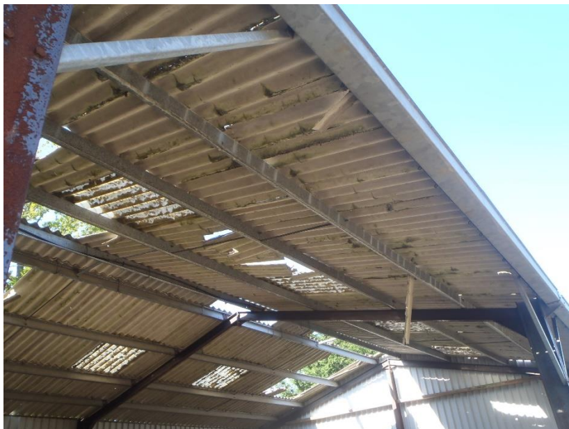
8. Barn Roof Damage
