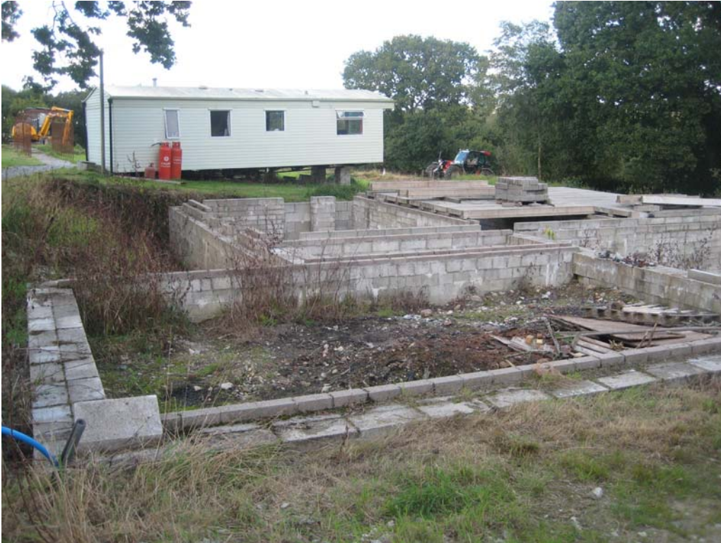
Proposed New House commenced in accordance with PA15/11460, groundworks, foundations, ground floor and drainage in place
