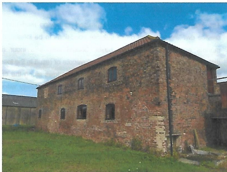
Photograph 2: Exterior view of the barn's masonry showing minor spalling
