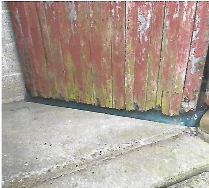
Photograph 9: Bottom of door now concealed with plastic sheeting
