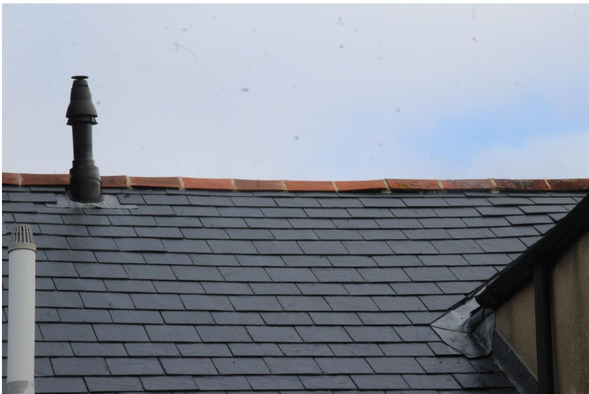
3. New roof with well pointed roof, but one raised ridge tile.
