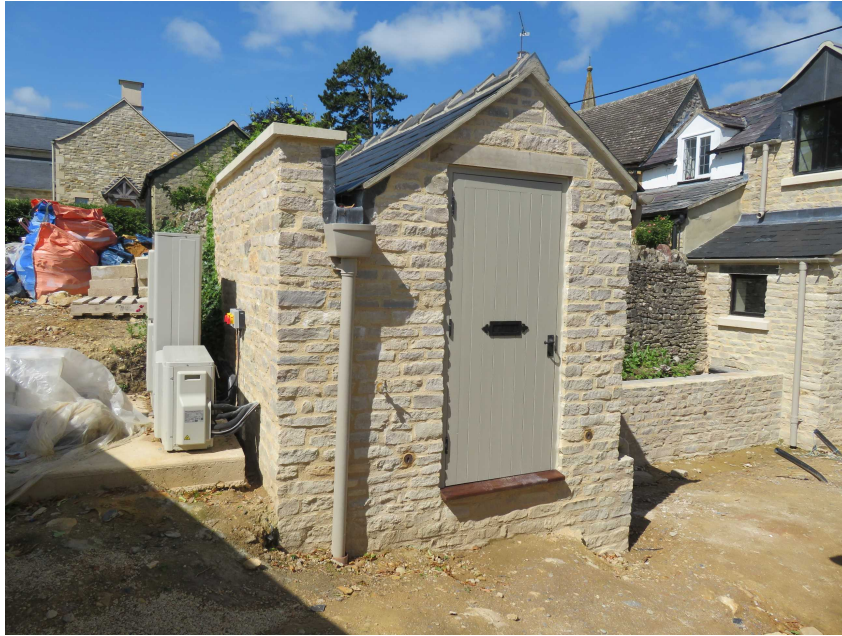
AIR SOURCE HEAT PUMP AND AIR CONDITIONING UNIT BEHIND OUTBUILDING VIEW 3
