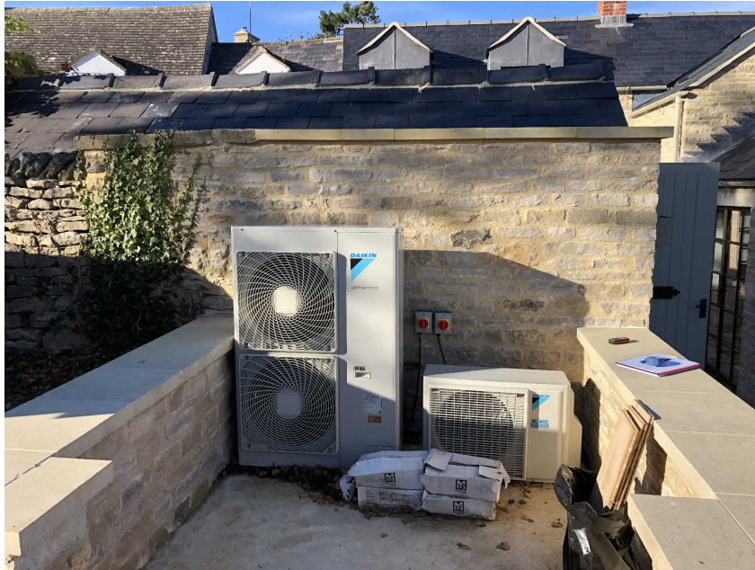
AIR SOURCE HEAT PUMP AND AIR CONDITIONING UNIT VIEW 1
