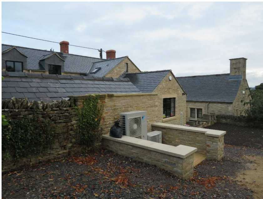
AIR SOURCE HEAT PUMP AND AIR CONDITIONING UNIT VIEW 2
