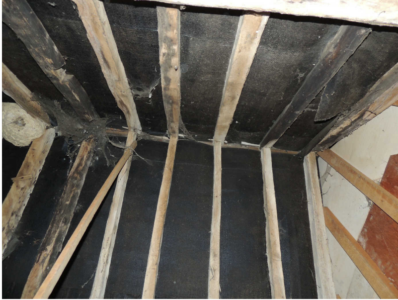
Photo 11: Note cobwebs in roof
