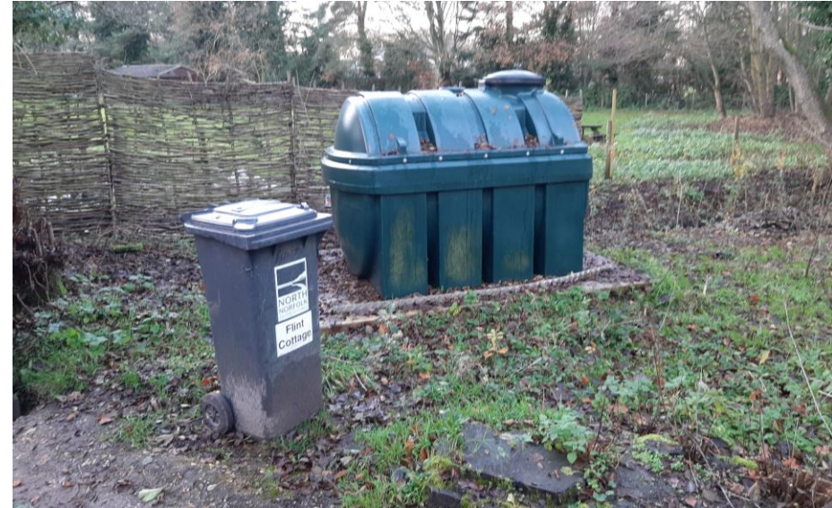
Plastic Bunded Oil Storage tank
