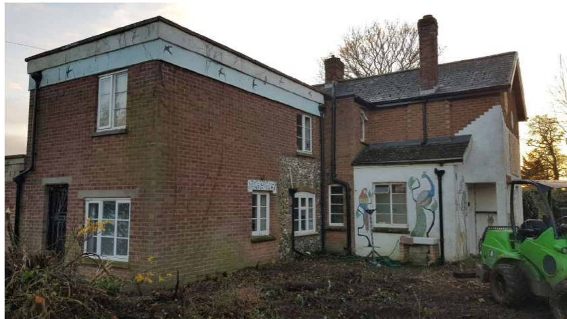
The rather unfortunate result of 20th Century development and alterations
