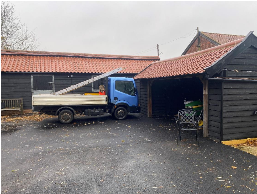
Photo 1: The building to be demolished is the open fronted structure on the right.
