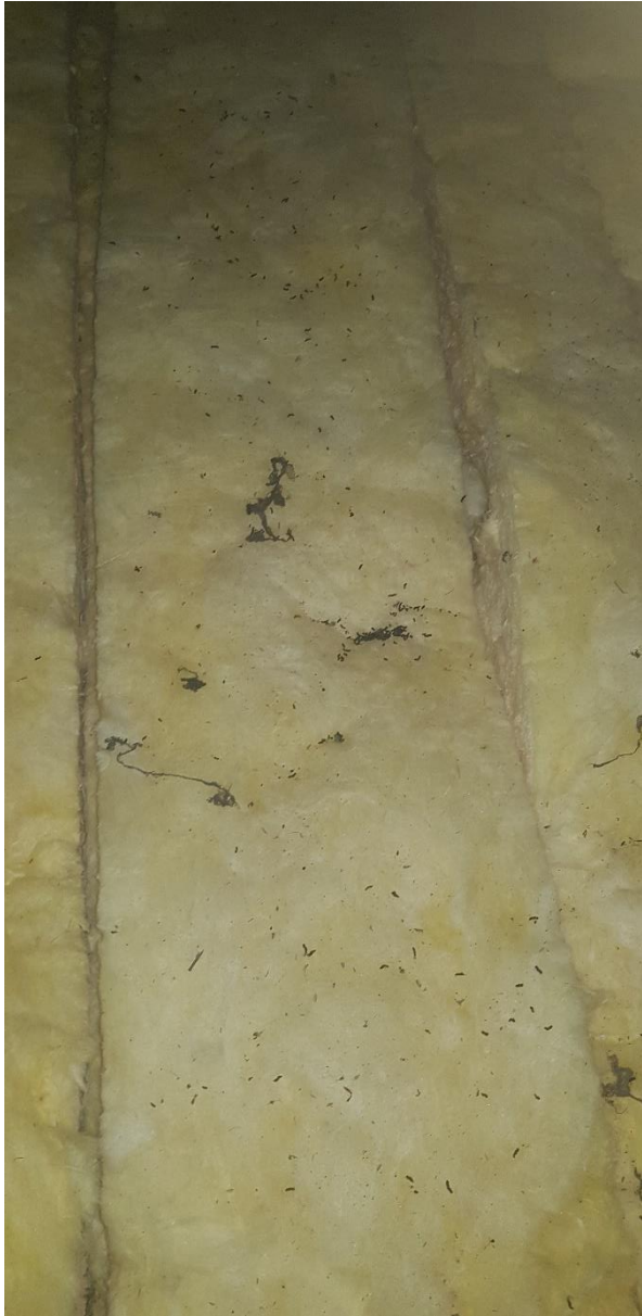
Picture 6: Showing the bat droppings on the insulation
