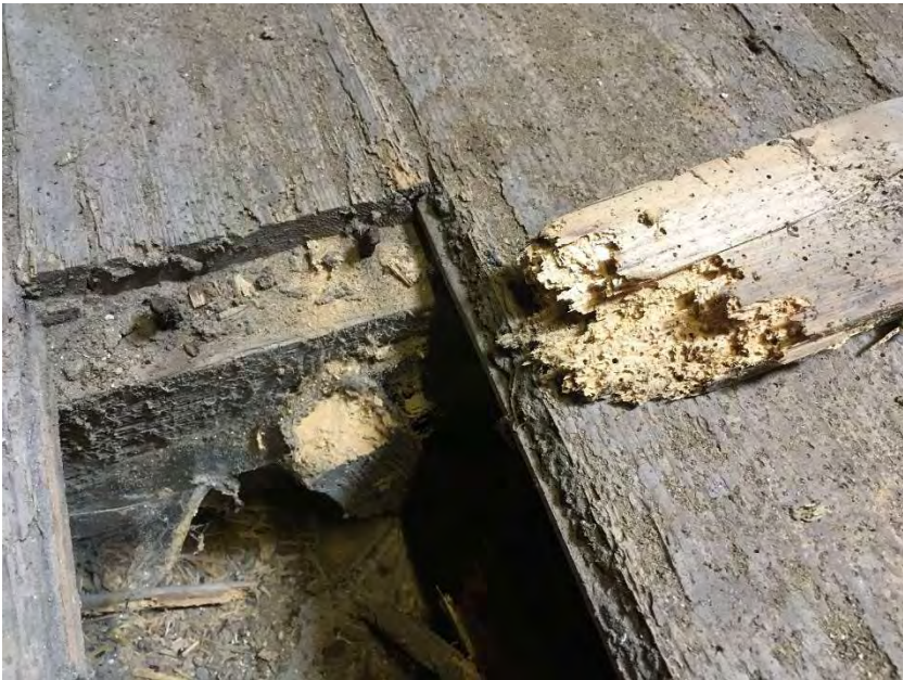
Photo 17 Close up of floor boards in former hayloft in fragile condition owing to woodworm infestation.
