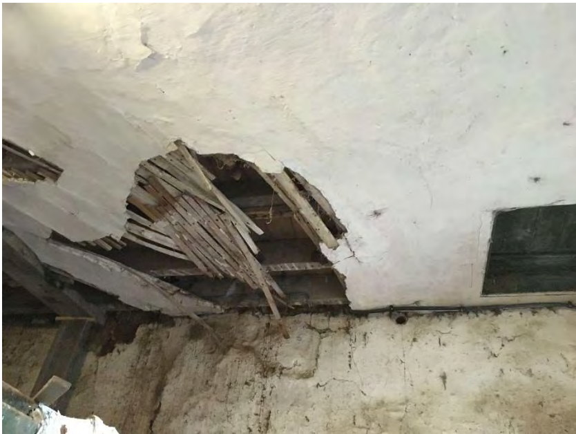
Photo 15 Internal view of damaged lath and plaster caused by water ingress through roof.
