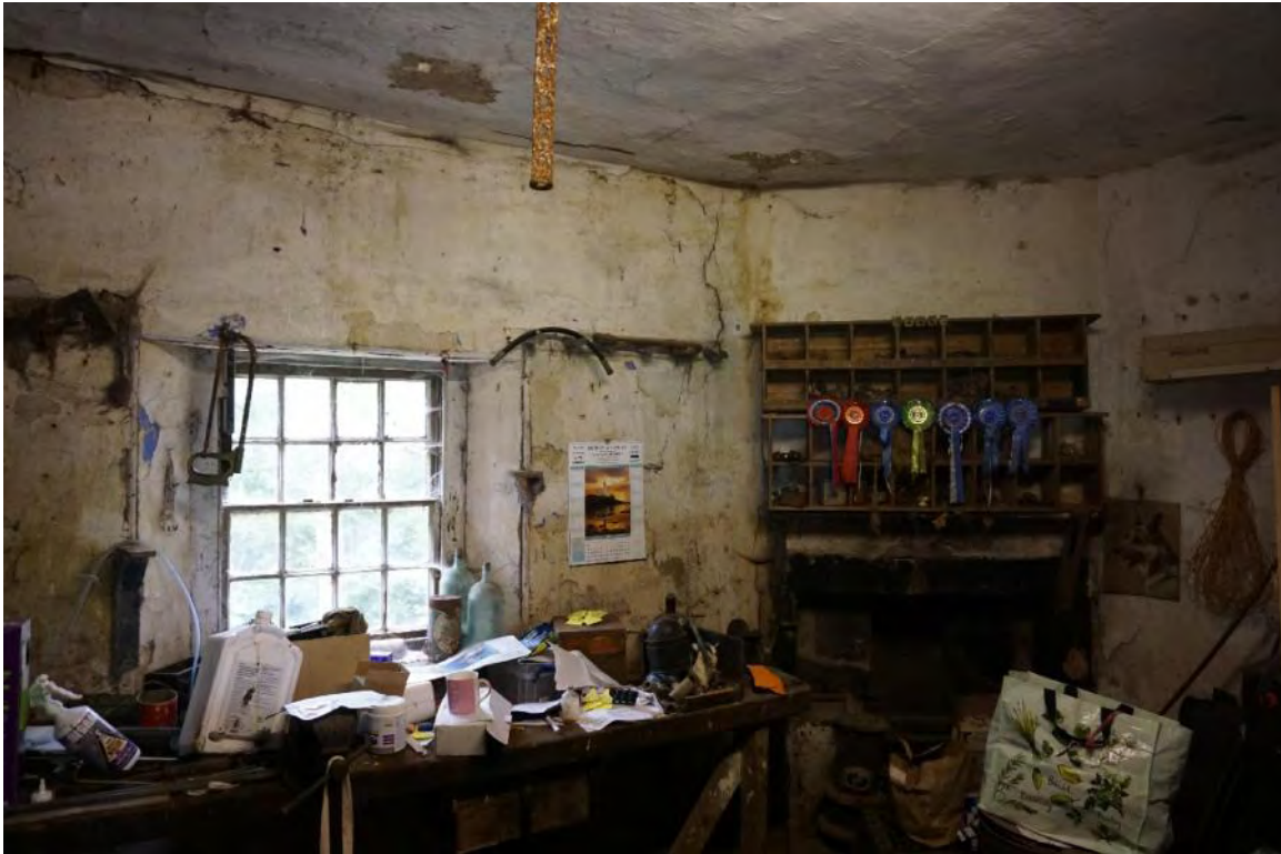
PHOTO 8 – Workroom between coachhouse and stable. – cracks to northwest corner
