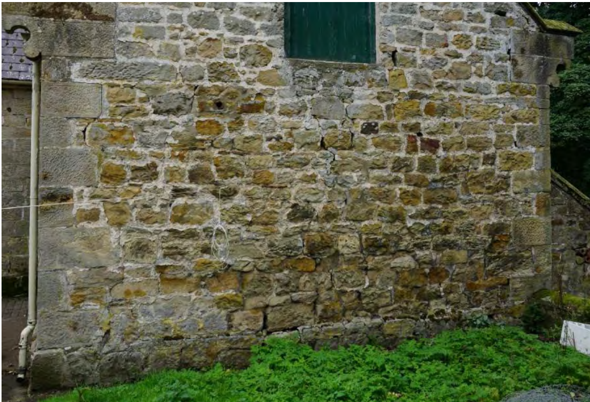
PHOTO 7 – Cracks to east gable – below hayloft door
