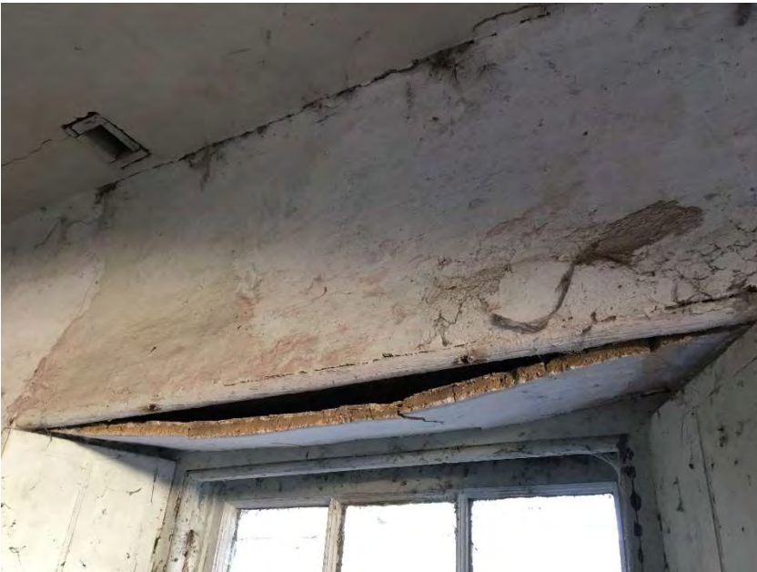
Photo 16 Internal view of damaged lath and plaster caused by water ingress over window.
