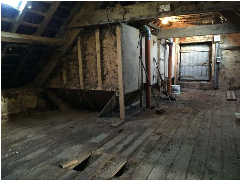
Photo 14 Internal view of former hayloft with 1960s feed hoppers and weak floor saturated after recent water ingress through slates.
