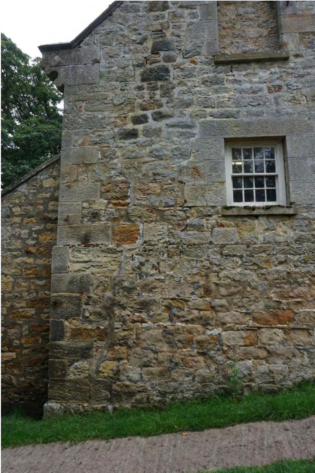
PHOTO 5 – Crack to northwest wall of main building (showing past repairs)
