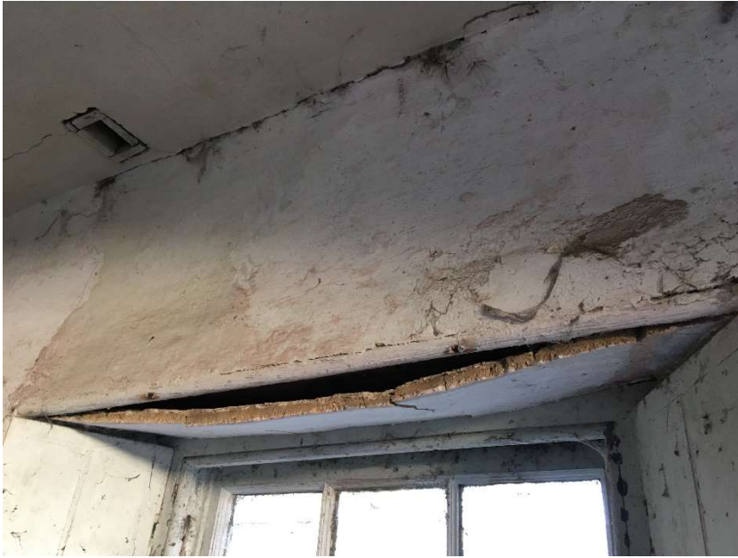
Photo 16 Internal view of damaged lath and plaster caused by water ingress over window.
