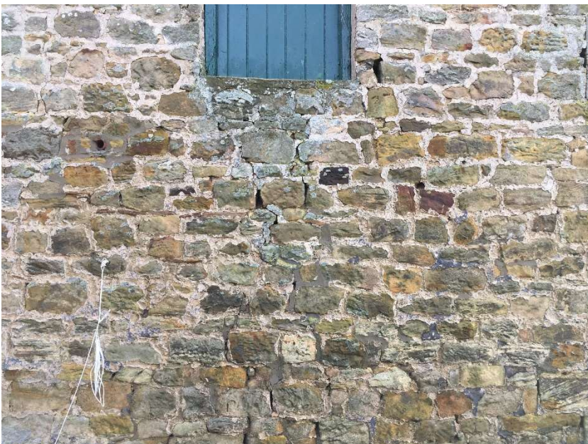
Photo 18 Close up of cracked masonry on east gable.
