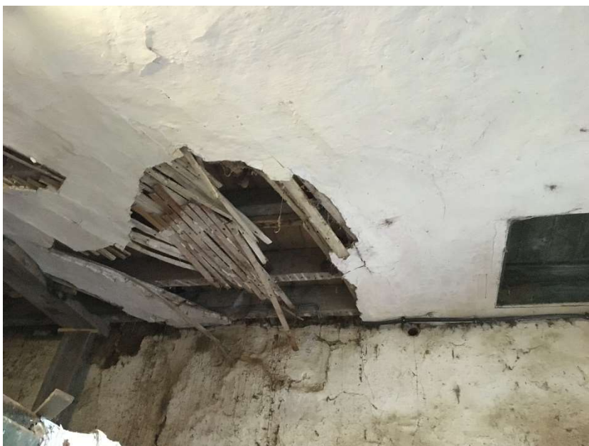
Photo 15 Internal view of damaged lath and plaster caused by water ingress through roof.
