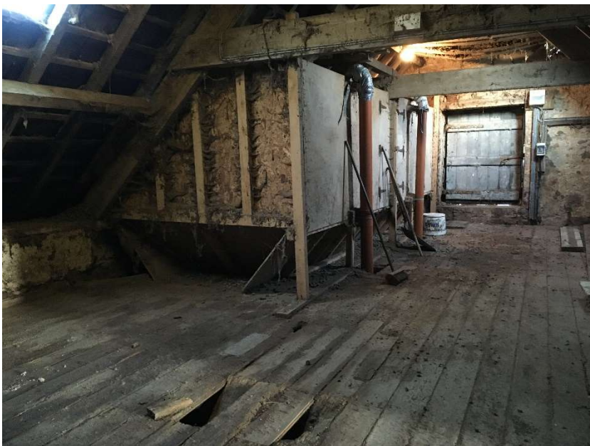
Photo 14 Internal view of former hayloft with 1960s feed hoppers and weak floor saturated after recent water ingress through slates.
