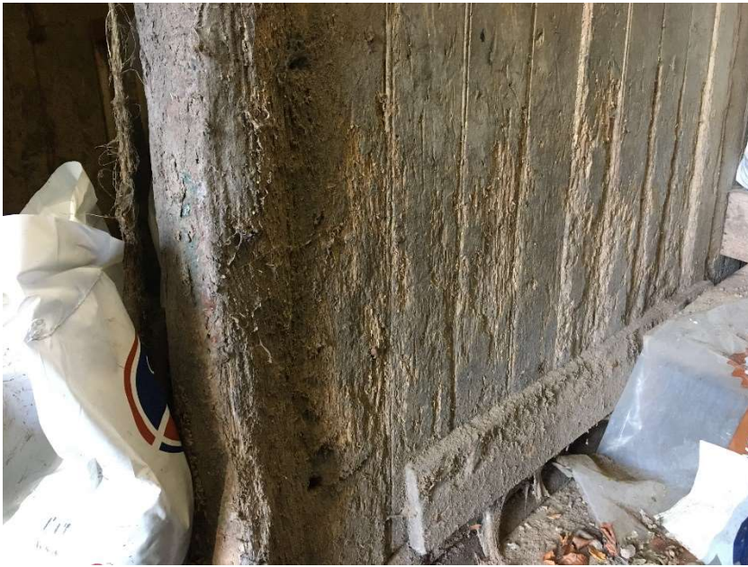
Photo 10 Internal view of stabling partition with chewed surface and woodworm infestation.
