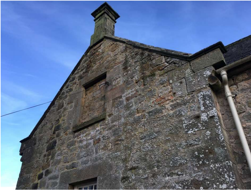
Photo 19 Close up of cracked and broken kneeler stone to west.
