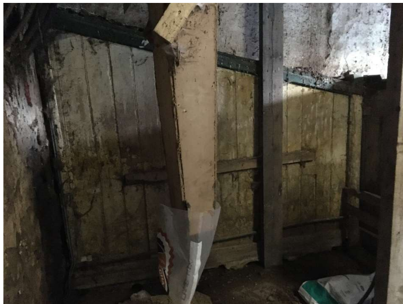
Photo 11 Internal view of former stable east end panel behind 1960s feed hopper.
