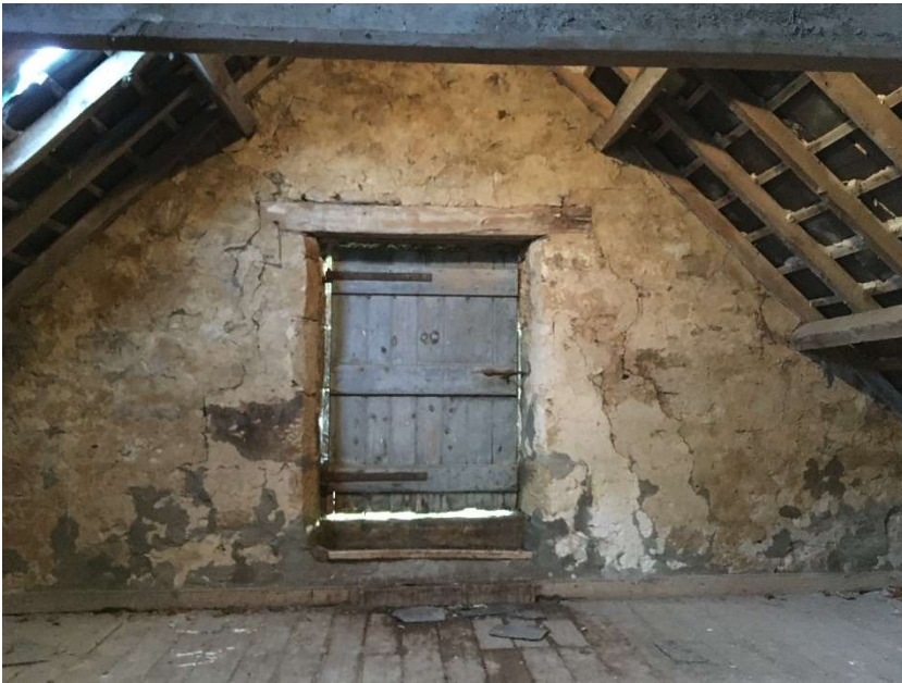
Photo 13 Internal view of hayloft with cracked masonry and wet floor after recent water ingress through slates.
