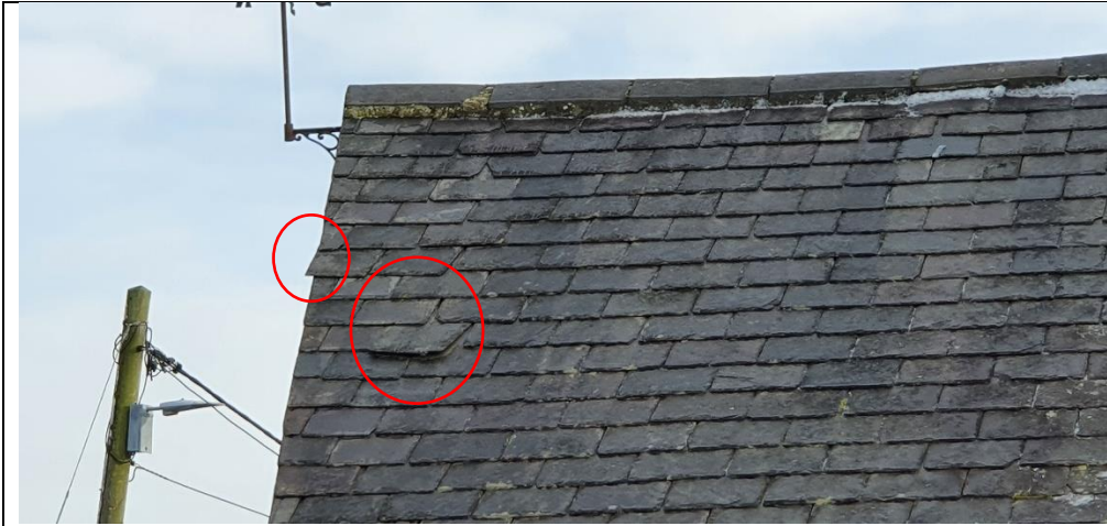
B1 slipped tiles (pictured above).
