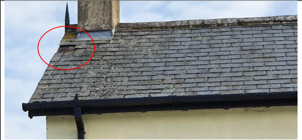
Missing tile on the main dwelling building which will not be impacted by the proposed development (pictured above).
