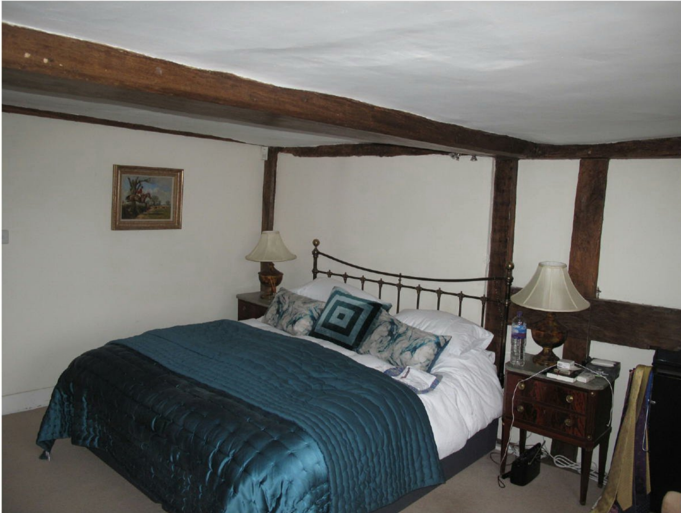
11. Timber beam in ceiling in line with truss in room S2, above, to be removed
