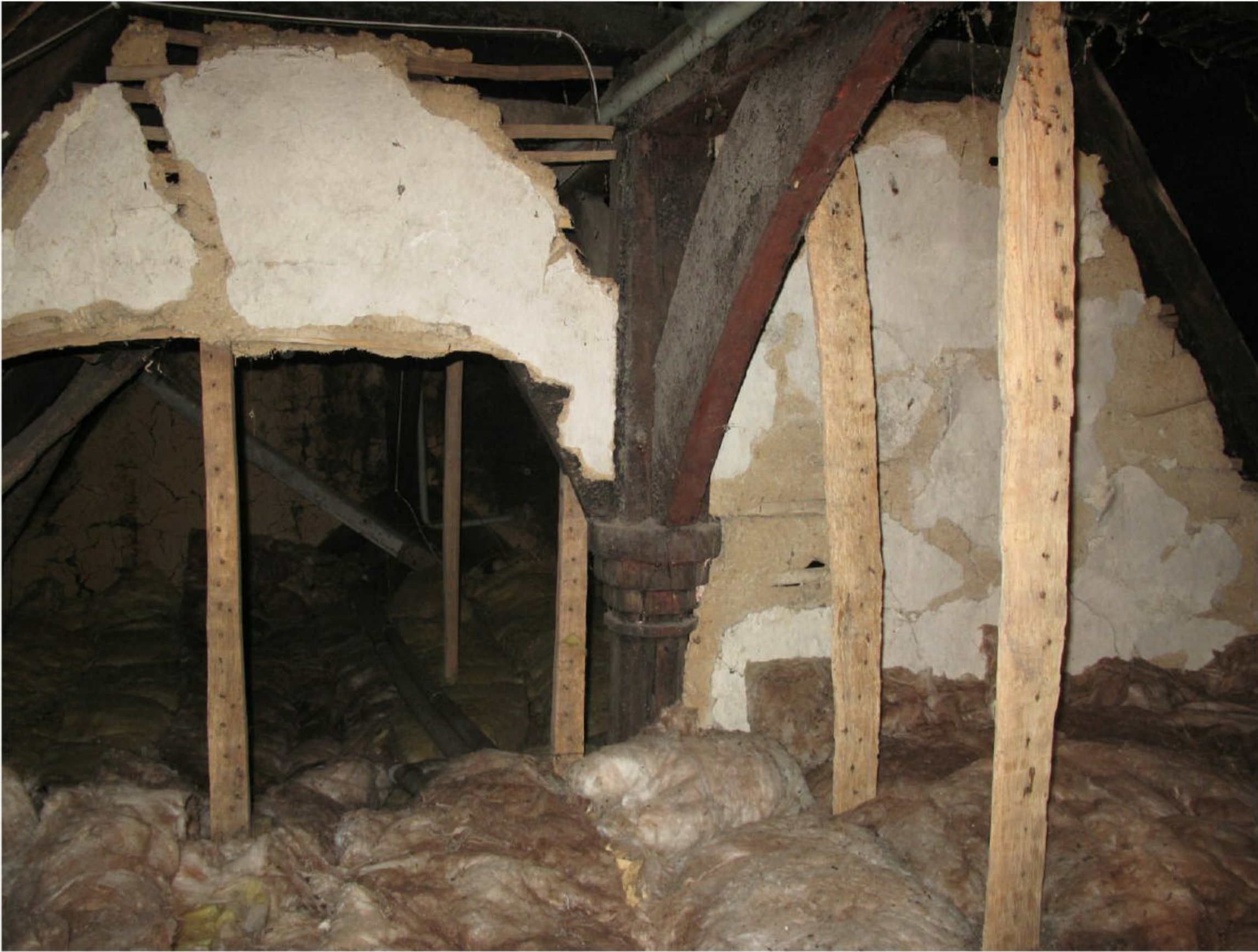
7. Roof structure to be repaired to allow props to be removed. Details to follow access after removal of insulation and ceiling finishes
