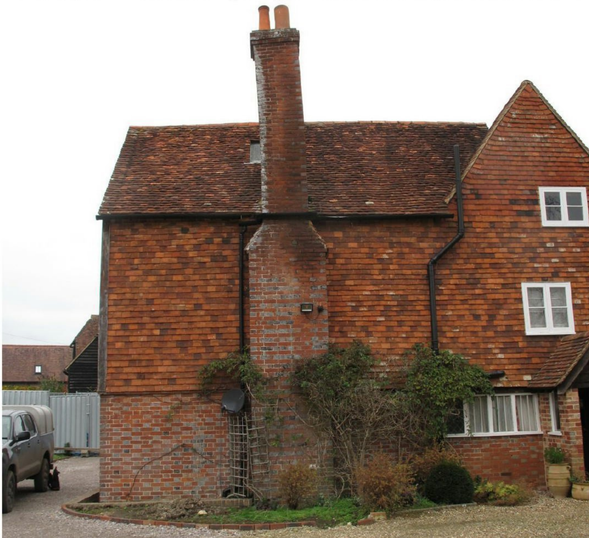
14. Chimney on east elevation leans towards the south
