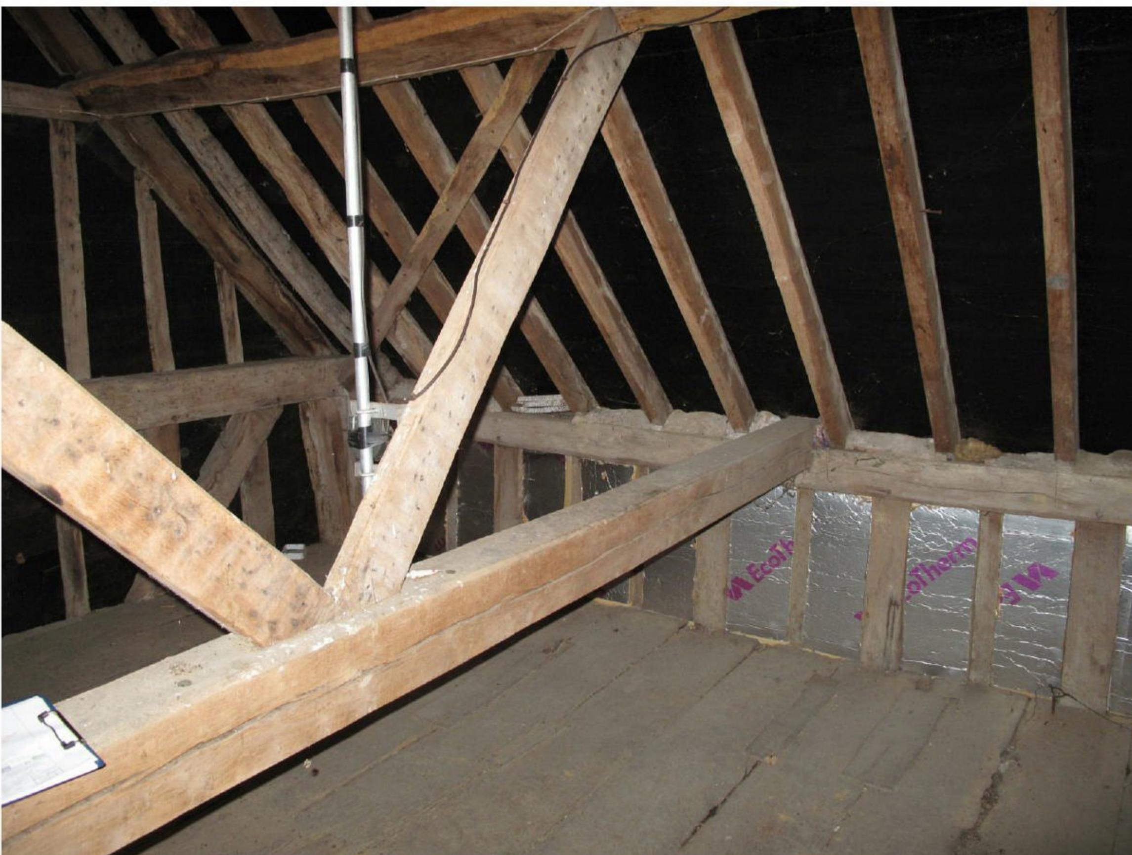
10. Room S2. Tie beam and raking props to purlins to be replaced with new structure
