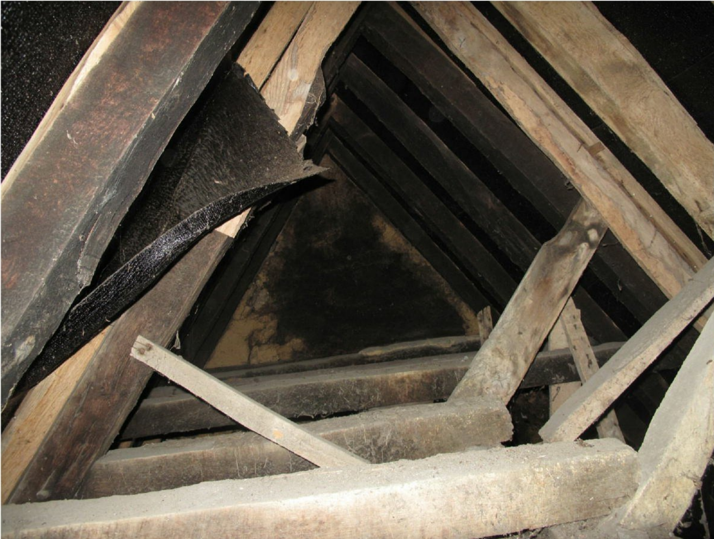
9. Extensive repairs needed to roof structure
