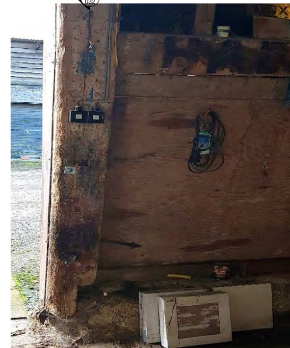
4 Post between bays 2&3 is inadequate (3.2.55*)
