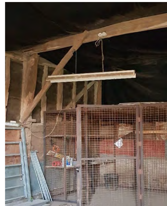
3 The principal post shows no connection to the tie beam and will need reinstating
