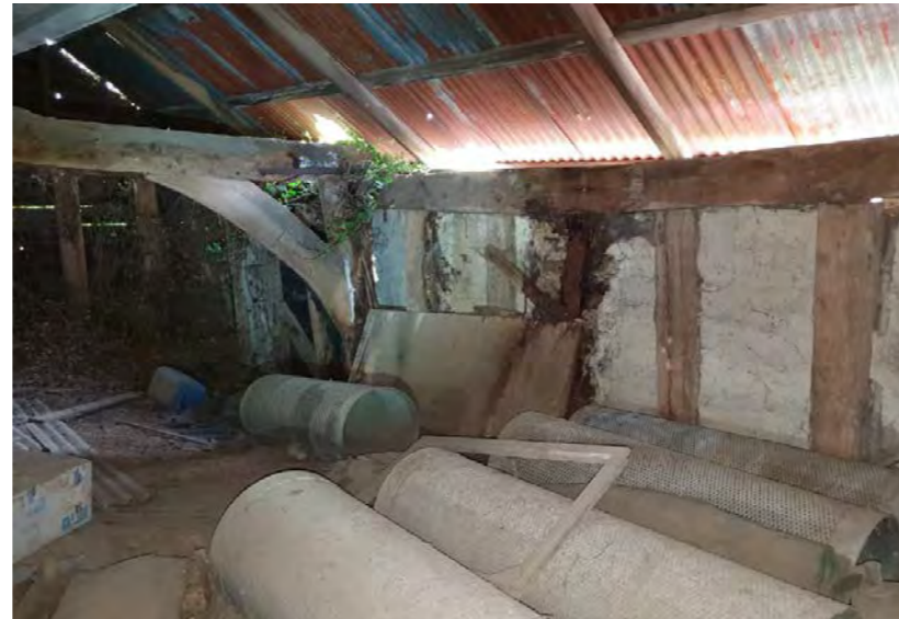
View 2: Looking west - timbers decayed at high level and water ingressed causing collapse of the lower section to SouthWest corner
