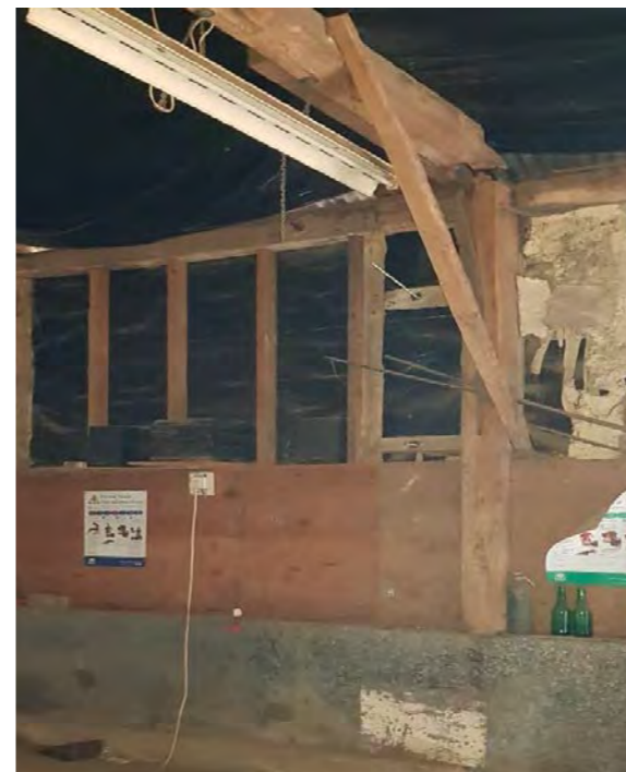
3 Timber post shows sign of decay and failure (3.2.73*)
