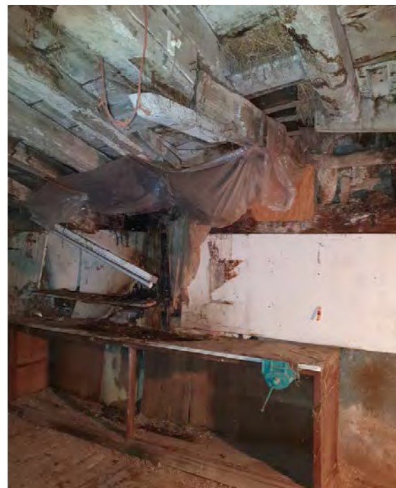
1 Timbers affected by the rainwater ingress, posts and studs deteriorated
