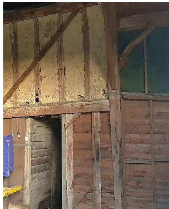
1 Historic post compromised - possible splice required (3.2.44*)
