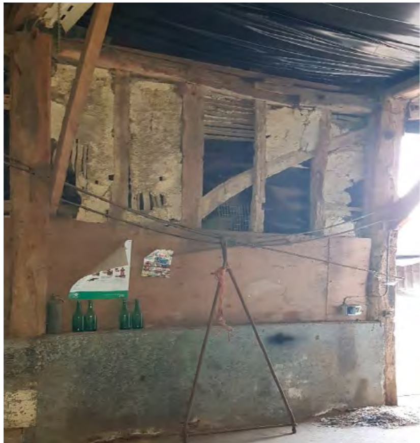
View 3: Looking west (Bay 4) - Timber post between bays 4&5 shows sign of decay and failure and it is not connected to tie beam
