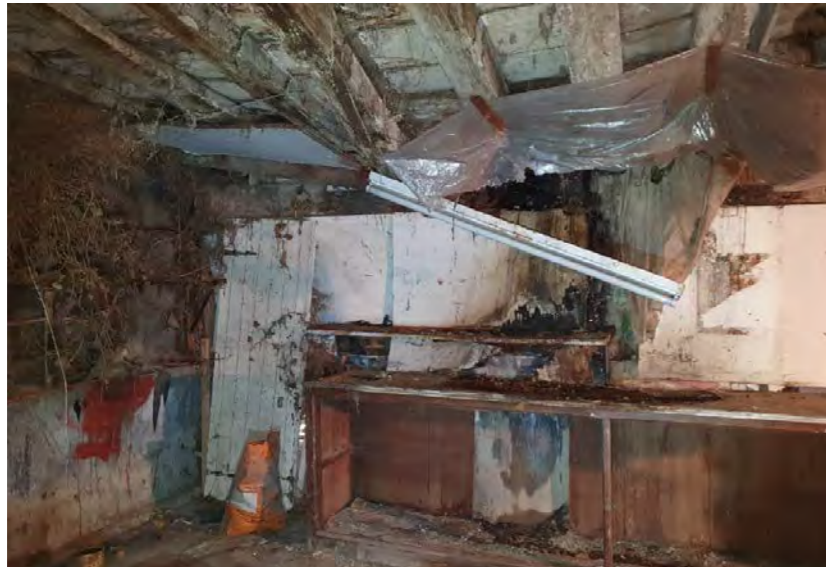
View 1: Looking southwest - Timbers been affected by rainwater ingress, studs and posts deteriorated (3.2.73*)
