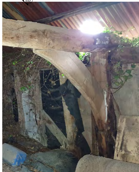
2 Timbers decayed at high level and water ingress causing collapse (3.2.82*)
