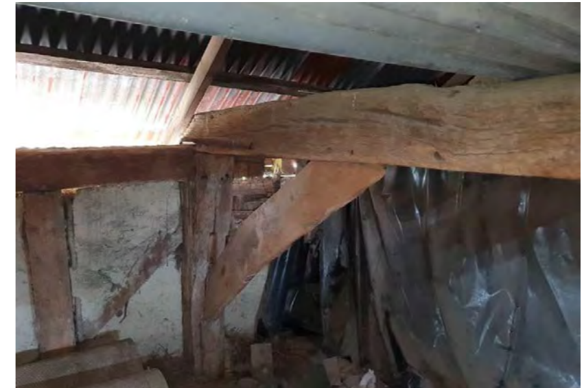
View 3: Looking east - elevation externally wrapped in a bituminous felt, studs and wall plates in reasonable good condition
