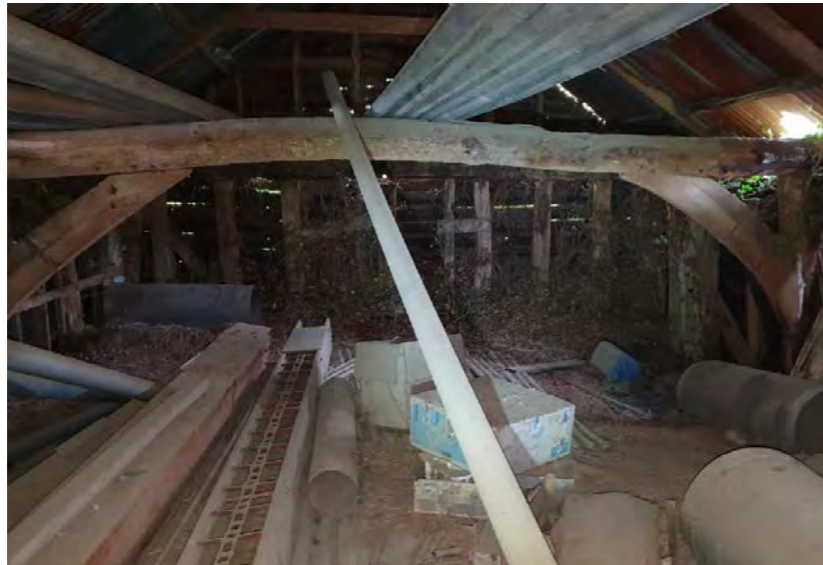
View 1: Looking south- vegetation growth throughout South facade
