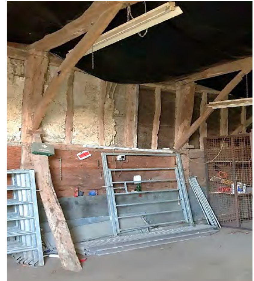
View 3: Looking east (Bay 5) - timber panels pulled out and replaced with sarking felt (3.2.50*)
