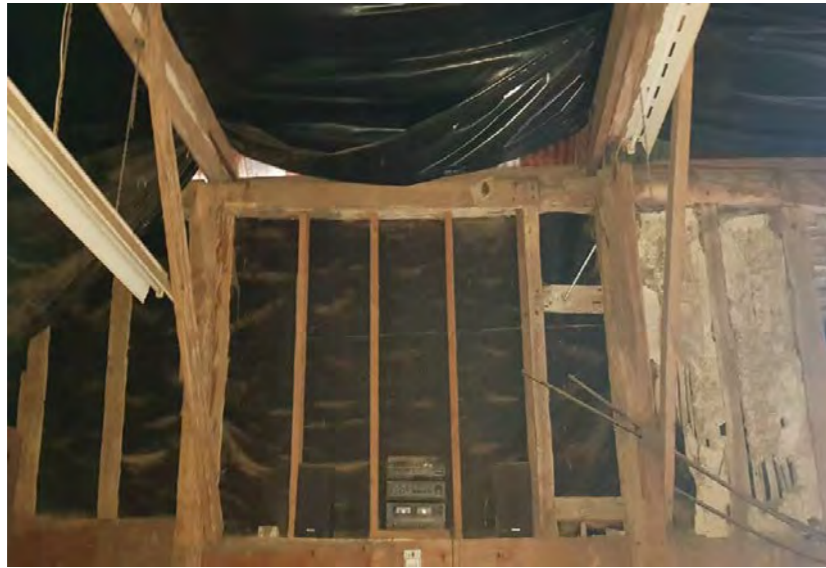
View 1: Looking west (Bay 5) - There is one original stud seen on the upper level, others replaced later (3.2.64*)
