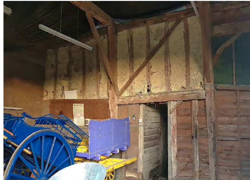
View 2: Looking east (Bay 1, 2 and 3) - historic studs, beams and mid rails seen on bays 1&2. Non-historic opening seen on bay 2 (3.2.37, 3.2.38, 3.2.39*)
