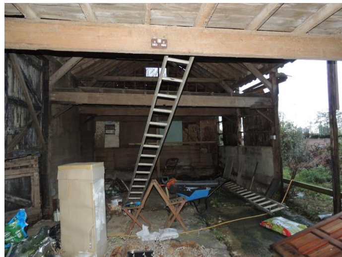
Photo 6: Looking south-westwards in barn. Note gaps in wall
