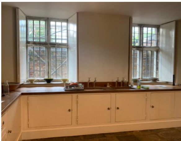
West wall of kitchen, showing the windows in question (WB3 and WB4). One casement in each window will open
