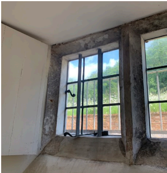
Window in basement room B1, with opening casement. We propose to replicate this detail for the opening lights in the kitchen
