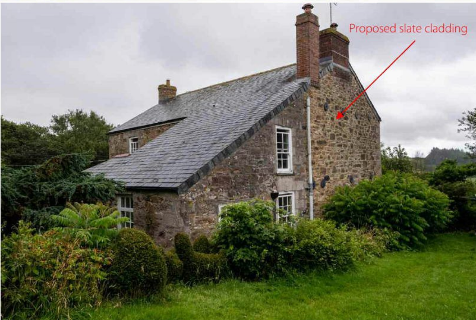
West elevation. Slate cladding is proposed to this elevation to address damp
