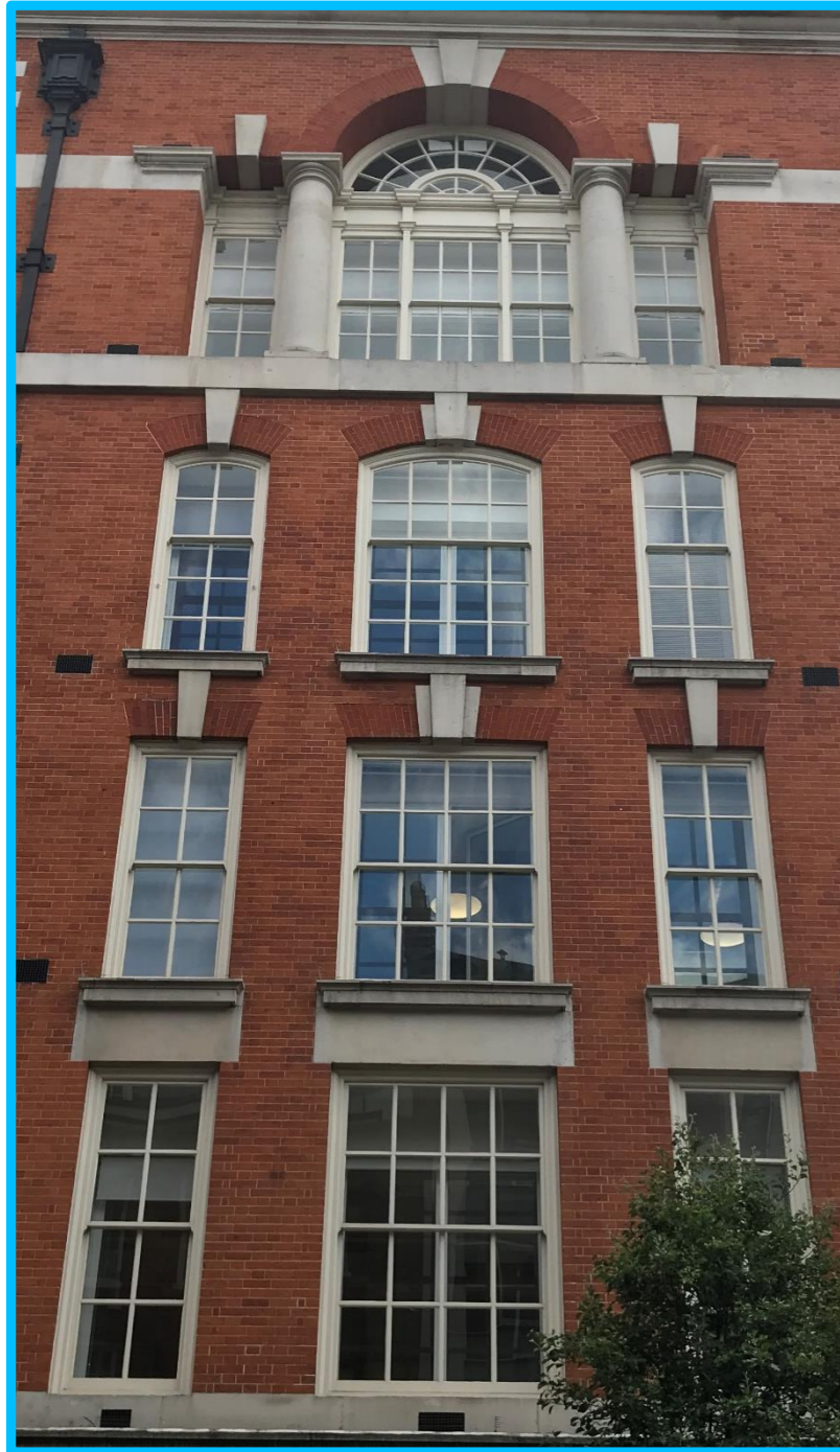
Above: cropped photograph of typical window types annotated in the adjacent elevation
