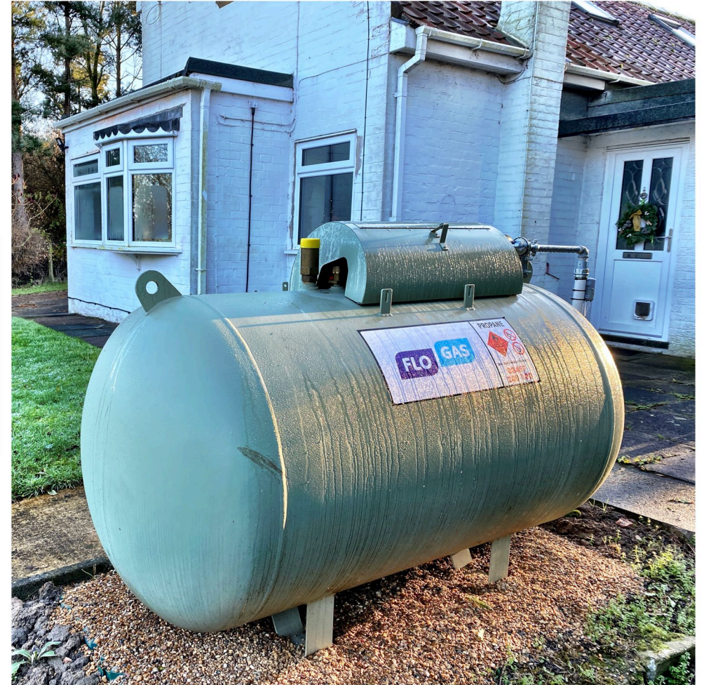
Road-side View of Installation
