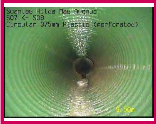
1, 00:00:49, 9.50 m Settled deposits, fine, 5% cross-sectional area loss
