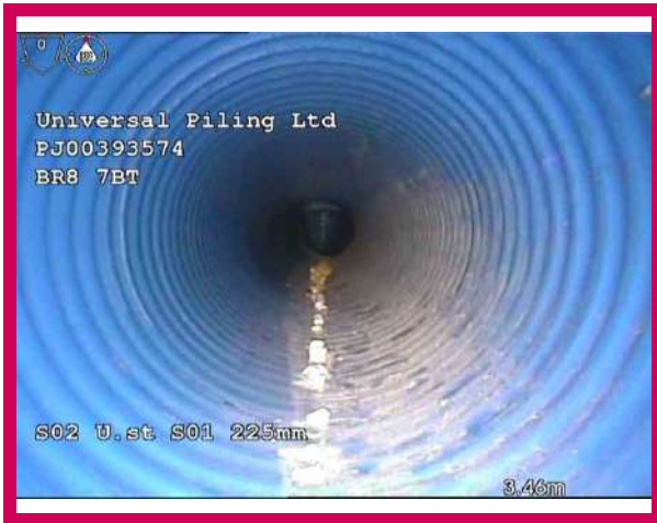
1, 00:00:19, 3.46 m Settled deposits, coarse, 5% cross-sectional area loss
