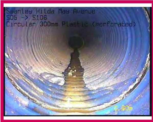
1, 00:00:01, 0.60 m Settled deposits, fine, 5% cross-sectional area loss, On pipe wall.
