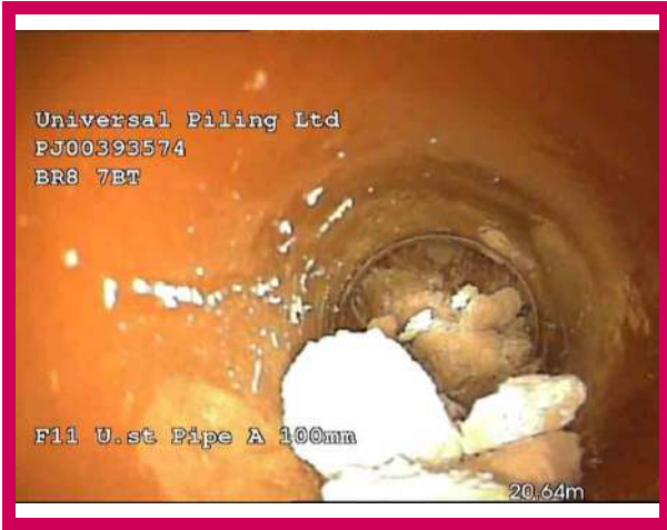
1, 00:01:05, 20.64 m Settled deposits, coarse, 30% cross-sectional area loss
