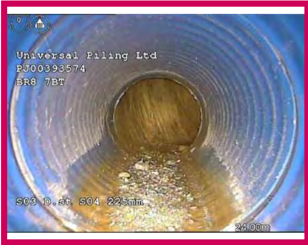
1, 00:01:58, 24.00 m Settled deposits, coarse, 5% cross-sectional area loss
