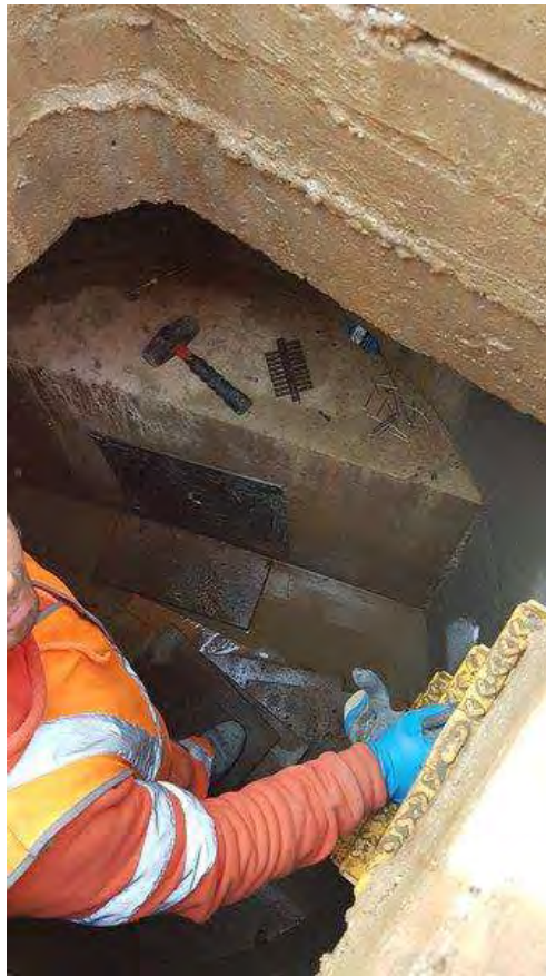
Fig D.1 – Orifice Plate Installation 1
