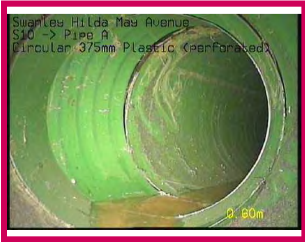
1, 00:00:02, 0.60 m Settled deposits, fine, 5% cross-sectional area loss, start
