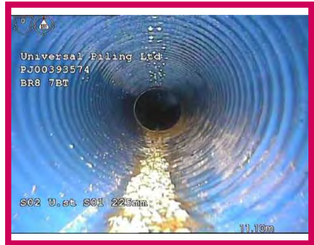
2, 00:00:58, 11.10 m Settled deposits, coarse, 5% cross-sectional area loss
