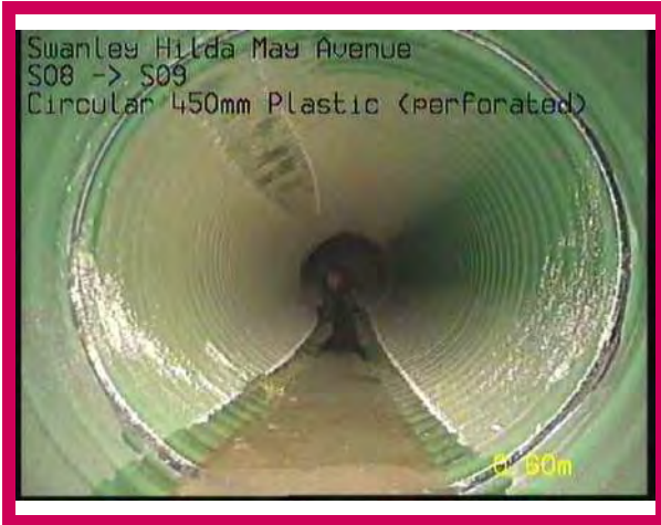
1, 00:00:02, 0.60 m Settled deposits, coarse, 5% cross-sectional area loss, start
