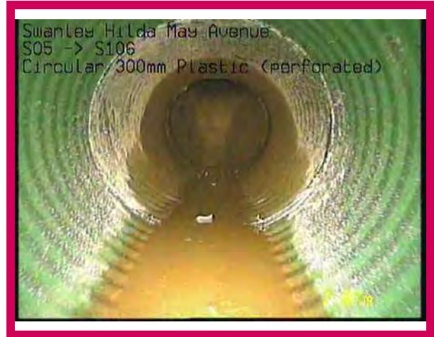
2, 00:00:31, 7.57 m Settled deposits, fine, 15% cross-sectional area loss
