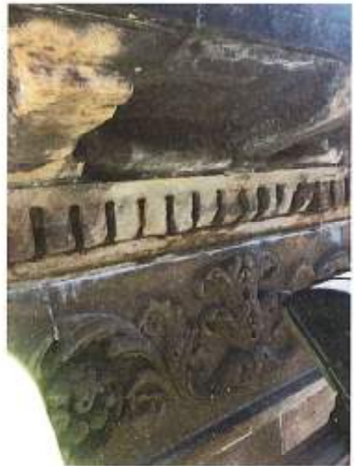
Fig 82: Friable dentil blocks (4 th floor projecting cornice)
