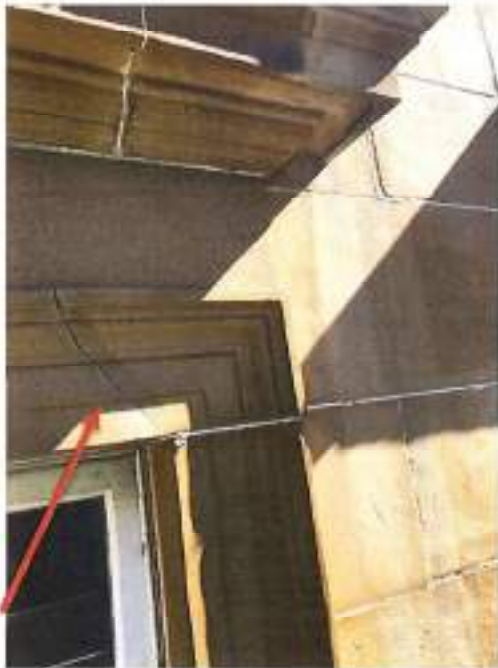
Fig 95: Cracked lintel 2 nd floor level
