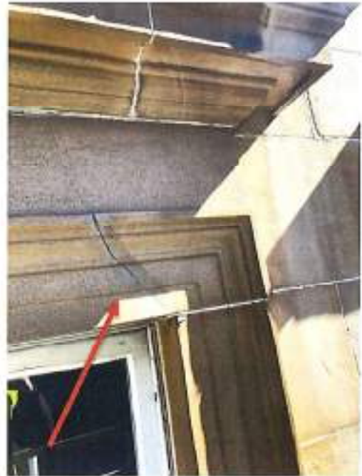
Fig 94: Cracked lintel 2 nd floor level
