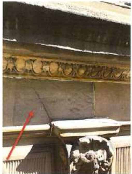
Fig 114: Crack ground floor level
