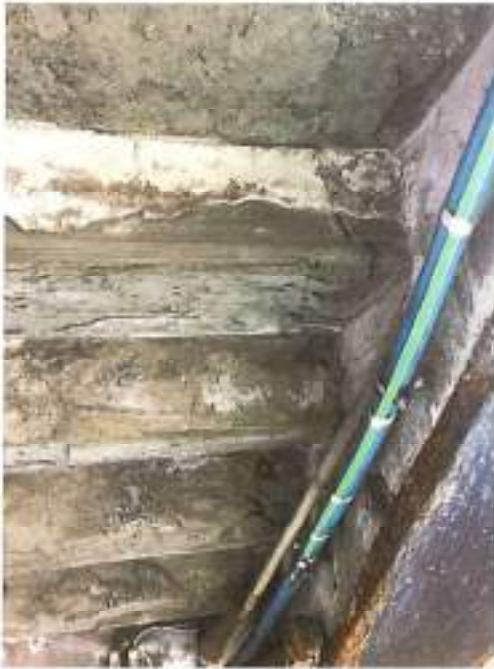
Fig 27: Underside of entrance steps
