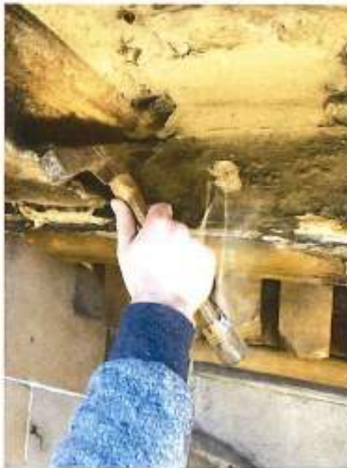
Fig 83: Friable stone under 4 th floor projecting cornice
