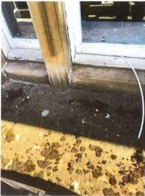
Fig 65: 4 th floor cill algae/moss
