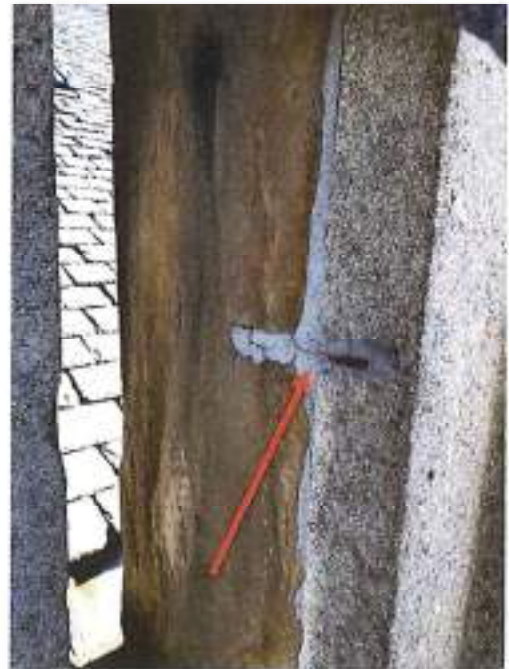
Fig 52: Corroded dowel in part concrete replacement
