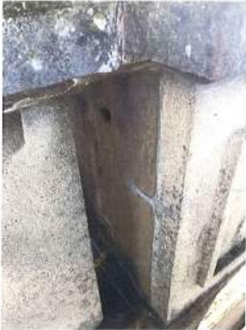
Fig 49: All part concrete replacement's ring boss
