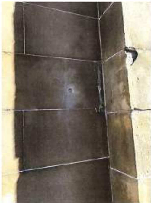
Fig 99: Area of spalling repairs 2 nd floor
