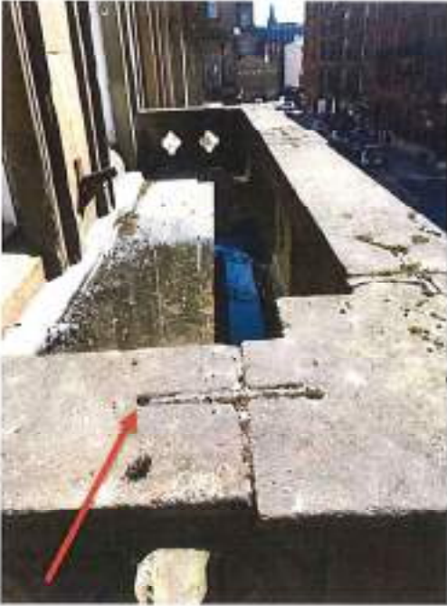
Fig 105: Corroded cramps parapet cope (Portico)
