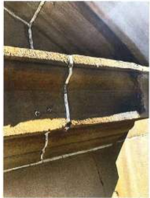
Fig 98: 2 nd floor hood pointing required
