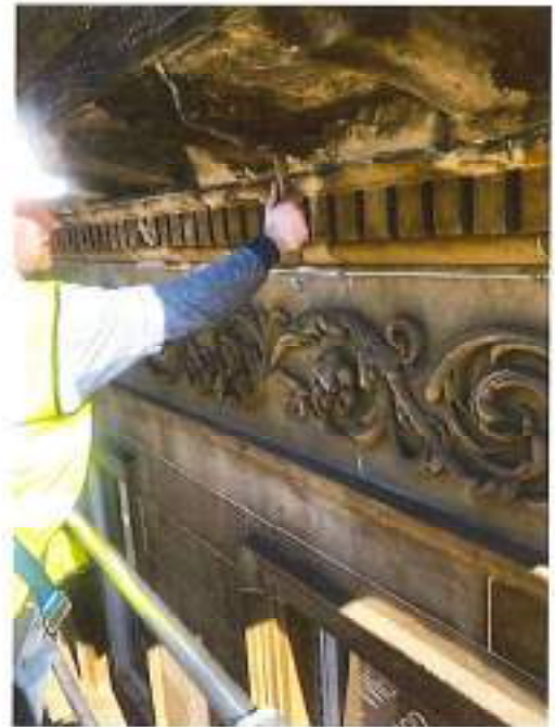
Fig 74: Underside of 4 th floor projecting cornice
