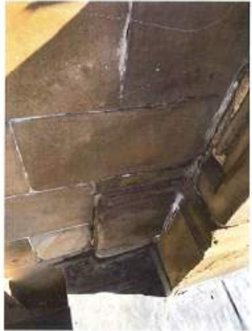
Fig 90: Area of pointing required 1 st floor level
