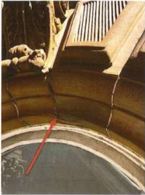
Fig 117: Ground floor window detail. (Spalling)
