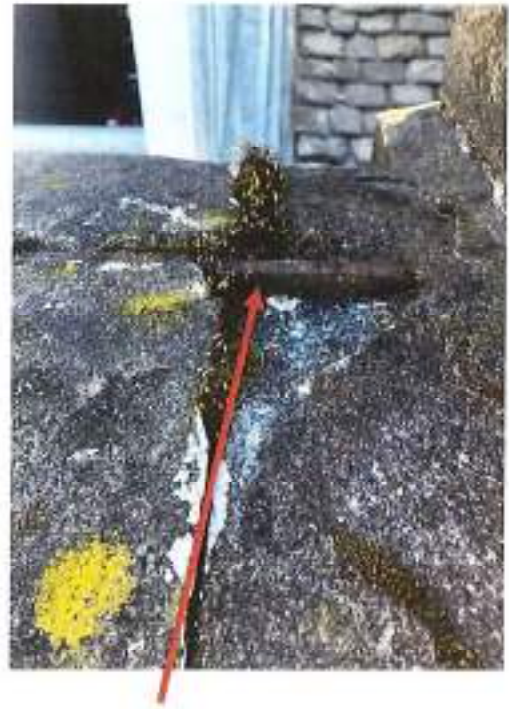
Fig 54: Corroded cramps in parapet copes
