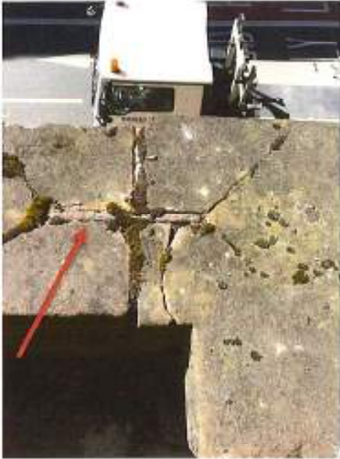
Fig 109: Corroded cramps parapet cope (Portico)
