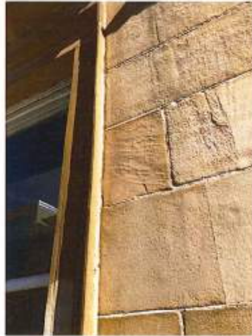
Fig 96: 2 nd floor pointing required
