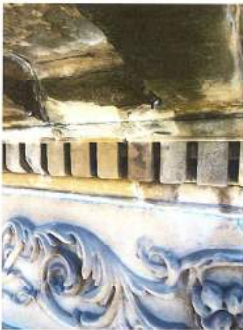
Fig 75: Underside of 4 th floor projecting cornice
