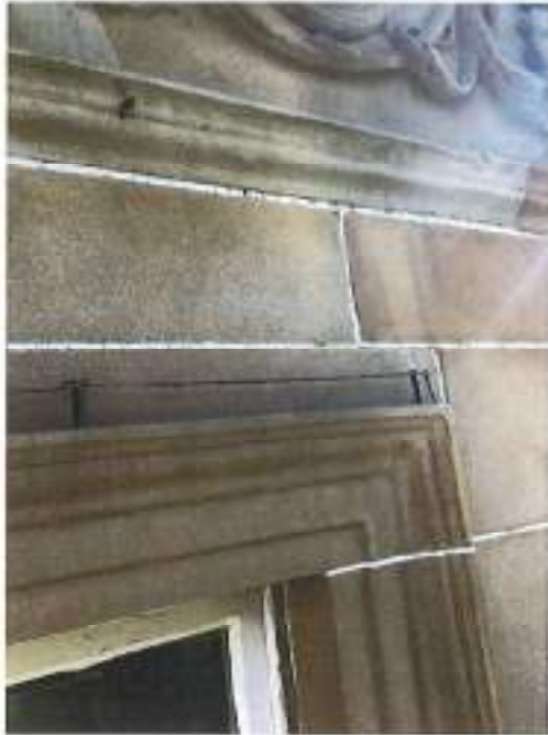
Fig 85: Bird deterrent spikes 3 rd floor windows
