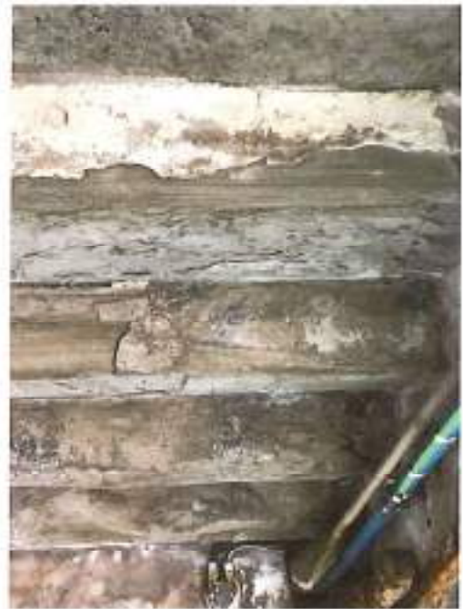
Fig 28: Underside of entrance steps
