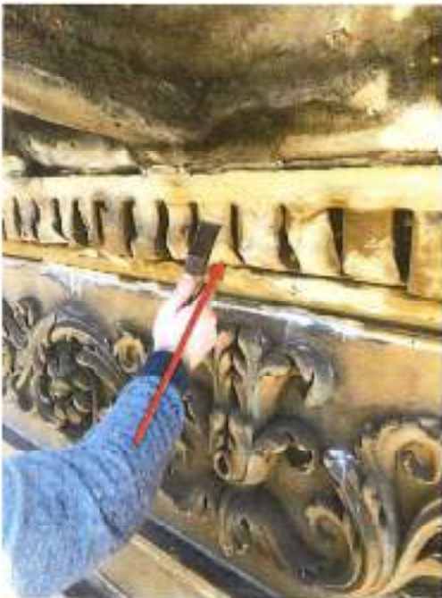
Fig 79: Friable dentil blocks (4 th floor projecting cornice)
