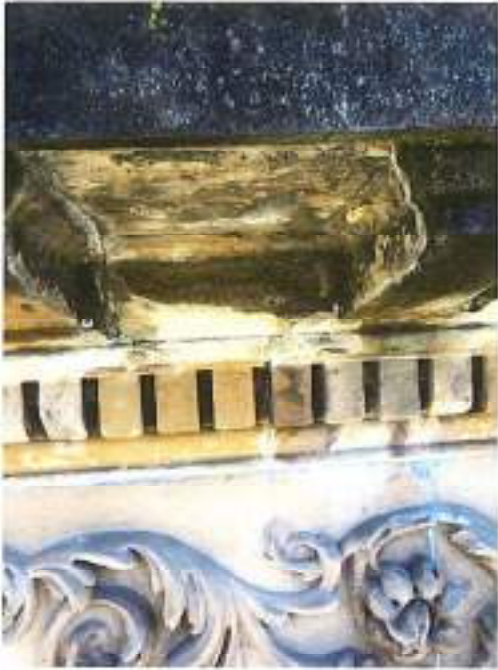
Fig 77: underside of 4 th floor projecting cornice
