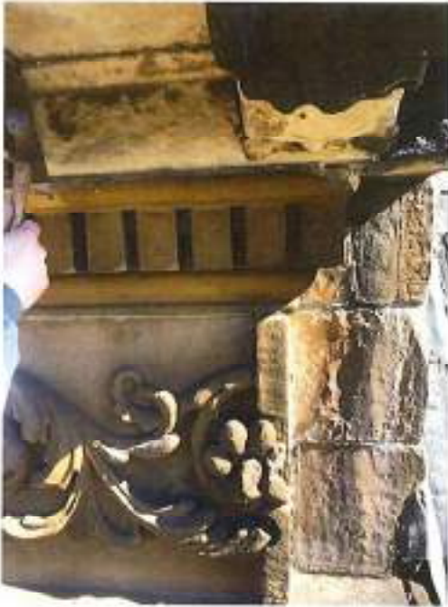
Fig 73: Underside of 4 th floor projecting cornice
