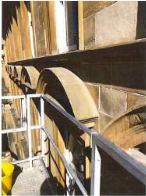
Fig 91: Overview of 2 nd floor hoods
