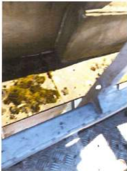
Fig 51: Algae/moss on eaves projecting cornice
