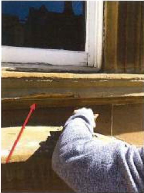
Fig 93: Friable cill 3 rd floor level
