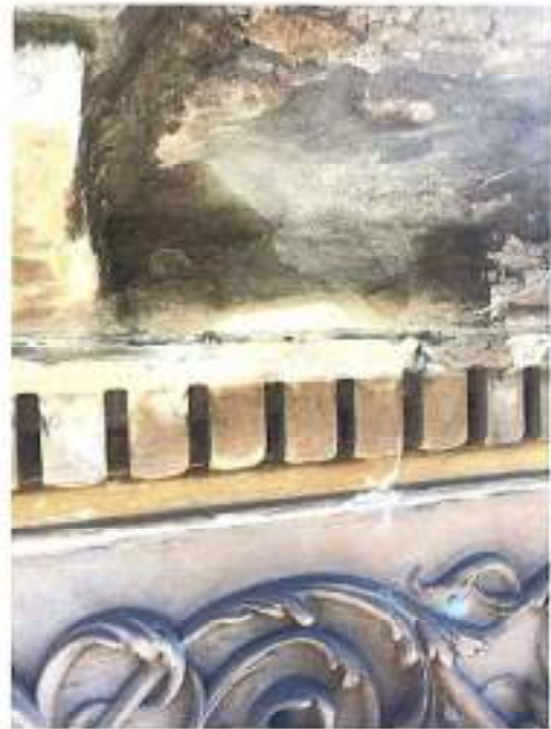
Fig 78: friable stone work
