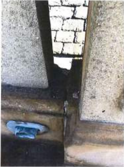
Fig 53: Open joints in parapet plinth course
