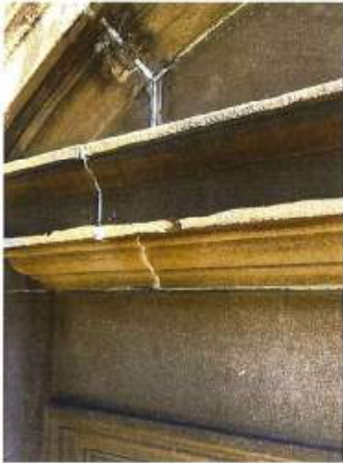
Fig 97: 2 nd floor hoods
