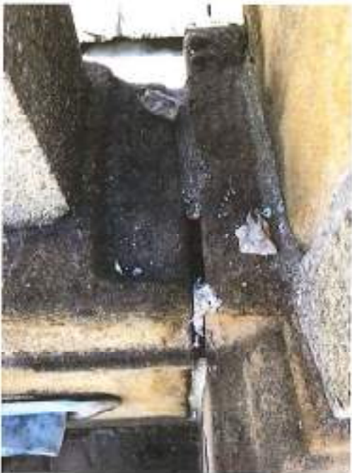
Fig 55: Open joints in parapet plinth course
