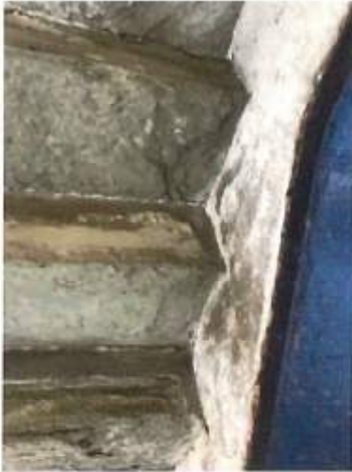
Fig 29: Underside of entrance steps
